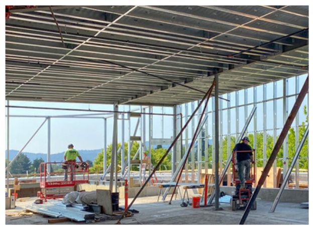
Below: Renovation of Oregon State University's Cordley Hall to Support Science and Engineering Departments.
