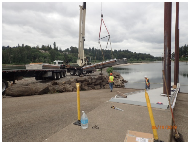
The recently-installed boarding dock at the Meldrum Bar boat ramp, operated by the City of Gladstone.
