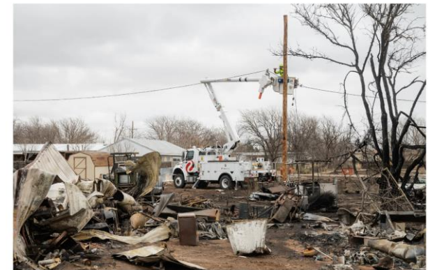
Workers replaced power lines that the Smokehouse Creek Fire damaged last month in Fritch, Texas. Desiree Rios for The New York Times
