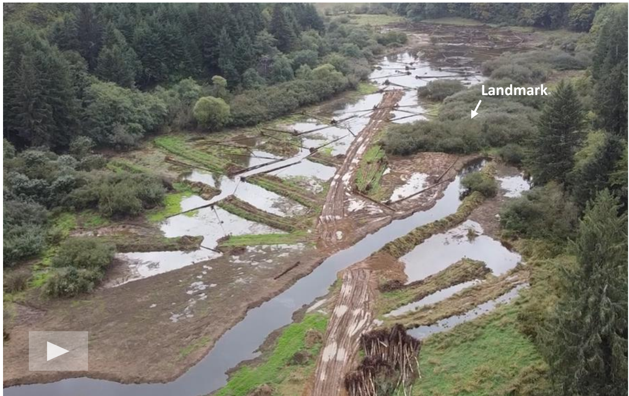
▲ Photo 3. Post-restoration conditions completed in 2023 by the Confederated Tribes of Siletz Indians along Fivemile Creek to increase channel complexity and floodplain connection, additional funds from OWEB were provided in 2024 to complete Phase 2 of this restoration project. Click on the image above to watch a short drone video of this restoration project area.
