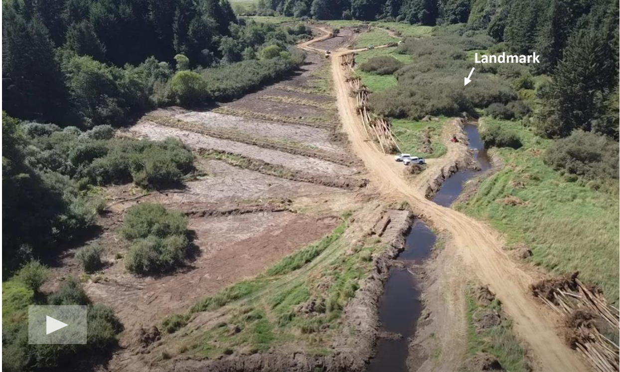
▲ Photo 2. During construction conditions along Fivemile Creek, located upstream of Tahkenitch Lake, Douglas County. Click on the image above to watch a short drone video of this restoration project area.
