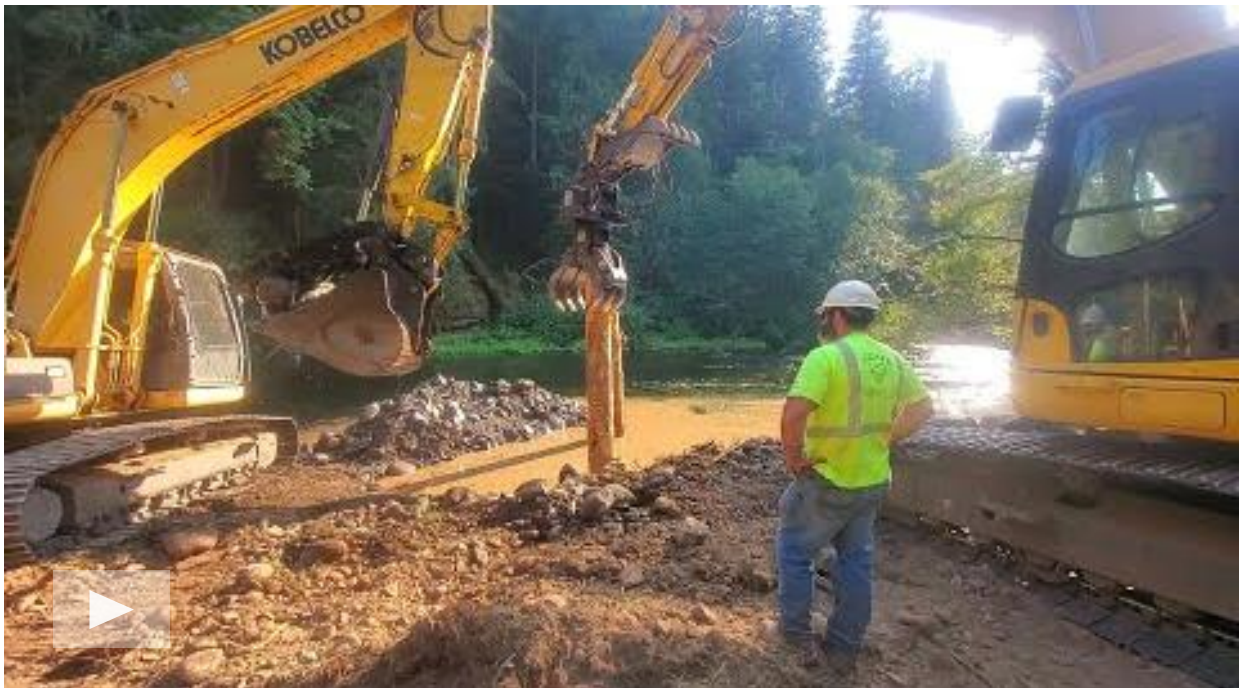
▲ Photo 8. Screenshot of large wood being placed in side channel of the Clackamas River on the Confederated Tribes of Warm Springs property. Click on the image above to watch a short video produced by the Clackamas River Basin Council to learn more about this collaborative project.
