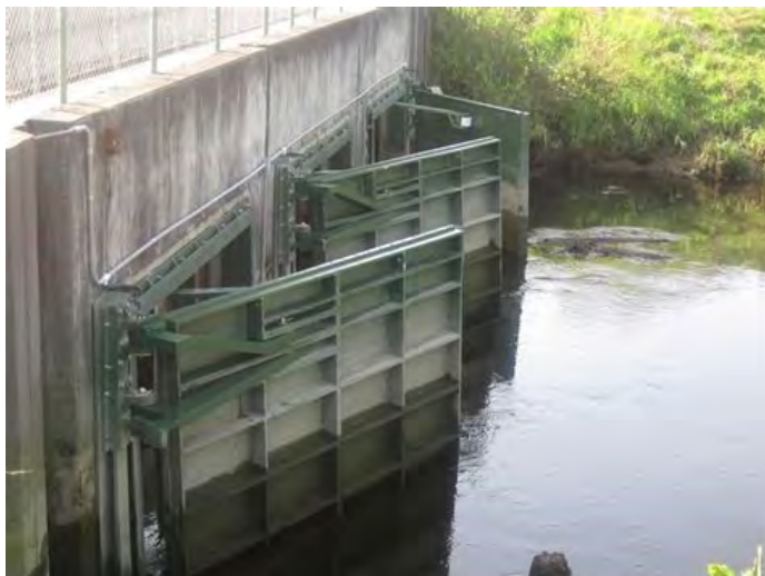
Replace existing tide gate with modern muted tidal regulator – two 10' wide by 8ft' tall gates with 7', 8',9',10' closure setting
