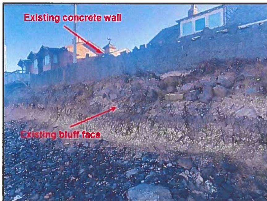
Photo 1: Existing eroded bluff face, and concrete wall at the top of the bluff.
