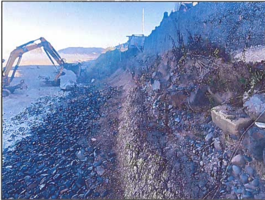
Photo 4: Looking northwest at the existing bluff slopes from the top of bluff.
