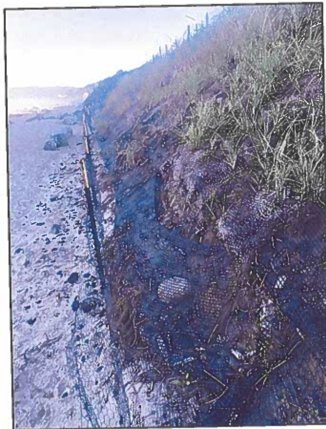
Photo 5. Looking north at the sand burrito-type SPS, installed in 2021 on the western edge of TL 2200. Note the substantial observed vegetation denuding and erosion that has occurred in the course of one winter season.
