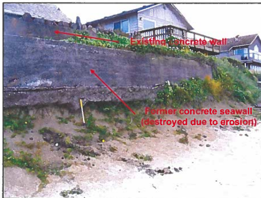
Photo 2: Undated photo of site beachfront and former seawall, presented in Witter et al (2009) as an “example of a seawall in Cannon Beach that has been undermined by wave erosion”.
