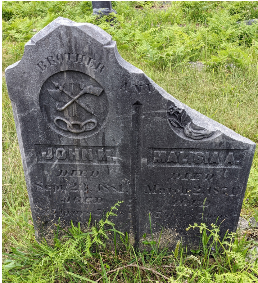
John & Malisia Bowron (B59-7): representative gravestone in need of new concrete base and resetting in mortar
