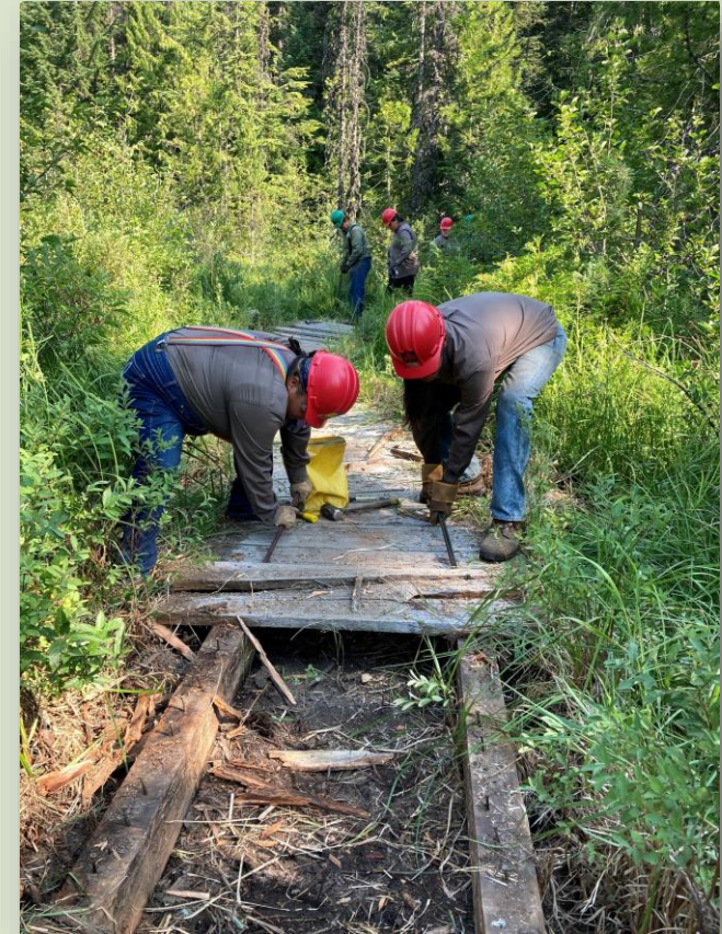
Northwest Youth Corps Tribal Stewards Crew, Trillium Lake boardwalk replacement, National Forest Foundation
