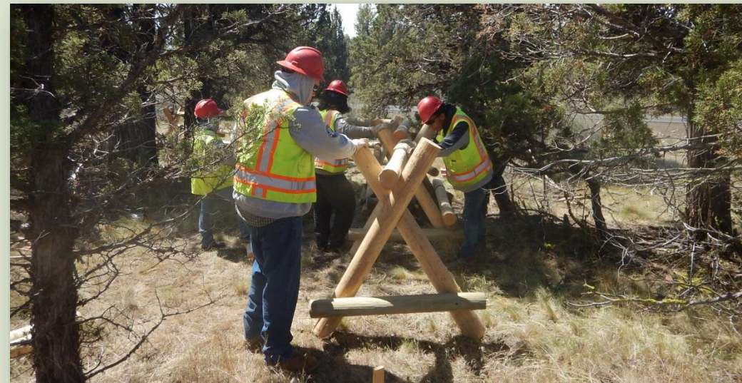
Heart of Oregon Youth Corps constructs fencing at BLM Prineville's Fryrear Trailhead
