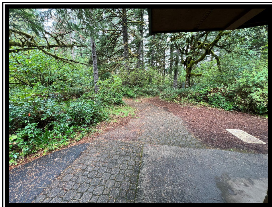
Figure 2 – Path to ADA site, uneven pavers.
