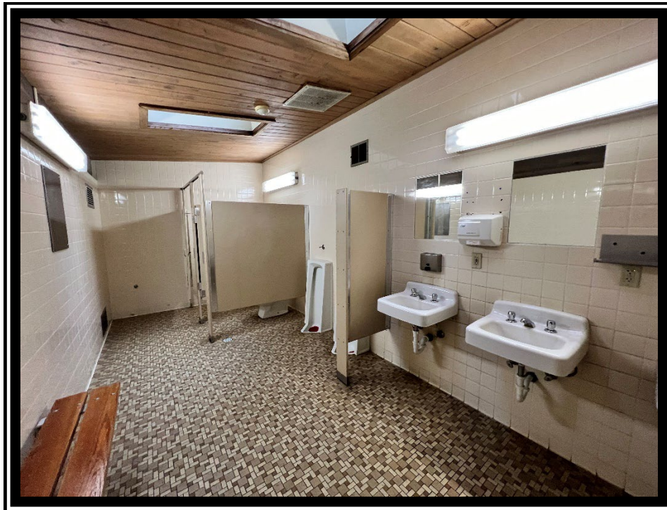
Figure 3 – Numerous repairs, difficult to maintain.
