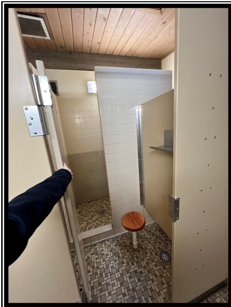
Figure 4 – Non-ADA showers, numerous partitions impede movement.
