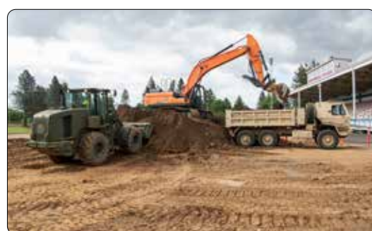
Photo by John Hughel, OMD Public Affairs ORARNG Soldiers assigned to the 1249th Engineer Battalion work to relocate over 8,500 cubic yards of soil, rocks and from the Centennial High School football field on May 23, 2023 during their two-weeks of IRT.
