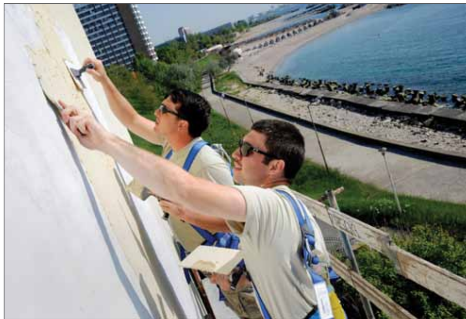
Tech. Sgt. Mathew Pixley and Senior Airman Daniel Beauchamp, from the 142nd Fighter Wing Civil Engineer Squadron, apply stucco to a medical clinic in the city of Mangalia, Romania, May 12. More than 30 Oregon Airmen traveled to Romania as a Deployment for Training (DFT) to assist with the Humanitarian Civic Assistance Program project.
