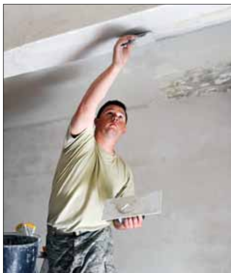
Tech. Sgt. Charles Jedda, from the 142nd Civil Engineer Squadron, applies plaster to upgrade and repair water damage to a health clinic in Mangalia, Romania, May 11.
