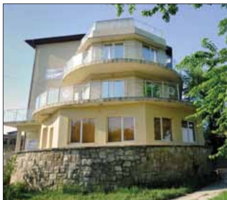
The Pavilion C medical clinic in Mangalia, Romania, was renovated with the help of the 142nd Fighter Wing Civil Engineer Squadron as part of EUCOM's Humanitarian Civic Assistance Program.
