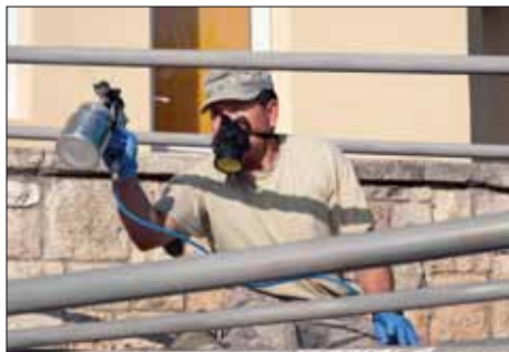
Tech. Sgt. Ramon Lopez, from the 142nd Civil Engineer Squadron, sprays paint primer prior to painting the handrails of a new wheelchair ramp at Pavilion C medical clinic in Mangalia, Romania, May 19.
