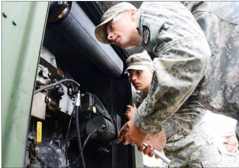
Spc. Corey Buoy and Spc. Franklin Dominguez, with the 3670 Maintenance Company ground support platoon, conduct preventive care and maintenance work on a military generator used by the City of Seaside as a back up power source in their water works section, Aug. 10.
