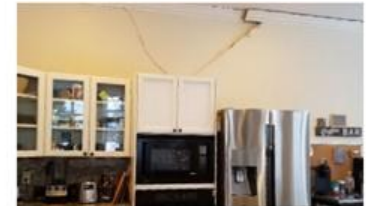
Significant cracking of wall finish materials. PHOTOS OF DAMAGE TO WALL FINISH MATERIALS FROM ANCHORAGE EARTHQUAKE. COURTESY OF JANISE RODGERS, AVAILABLE AT WWW.EERI.ORG, LAST ACCESSED 8/3/19
