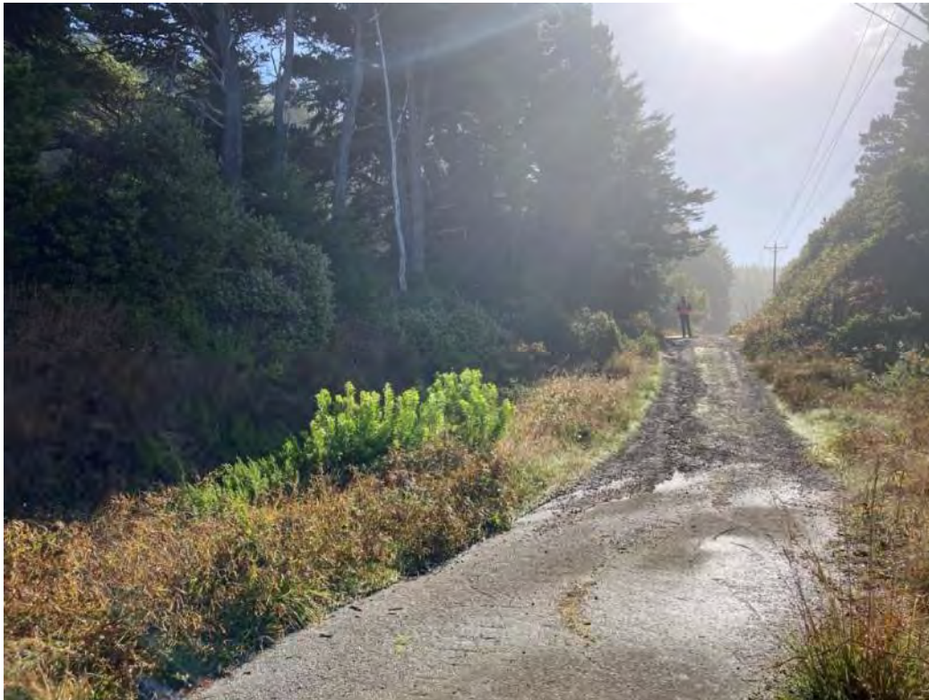
Exhibit 1: Vertical offset and pavement damage on Old US 101 along the southern margin of the slide.
