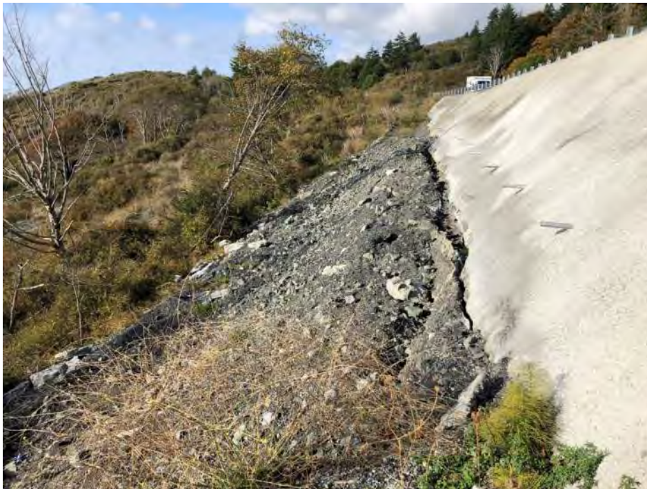
Exhibit 9: Localized failure of the slope below US 101 southbound. The failure caused damage to the existing soil nail stabilization including an approximate 1-foot gap at the bottom of the shotcrete facing.
