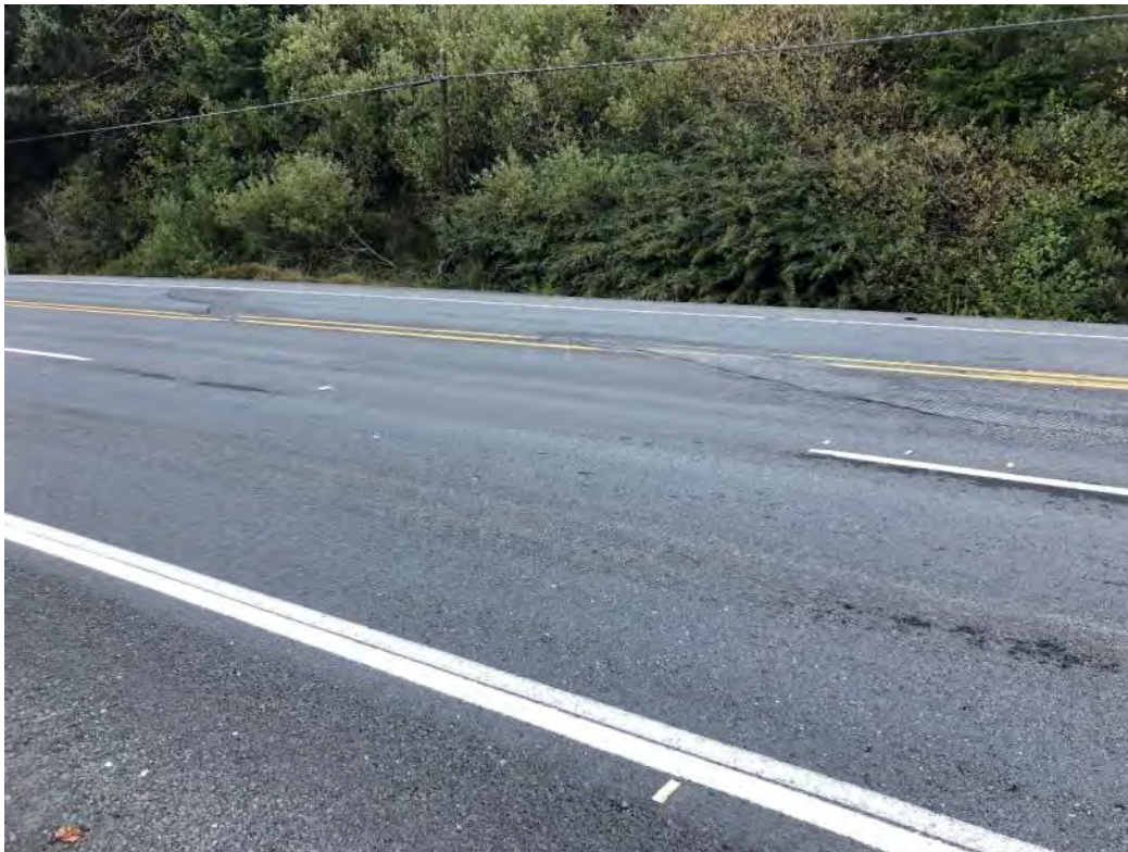
Exhibit 21: Tension cracks along south flank of slide running through all lanes of US 101
