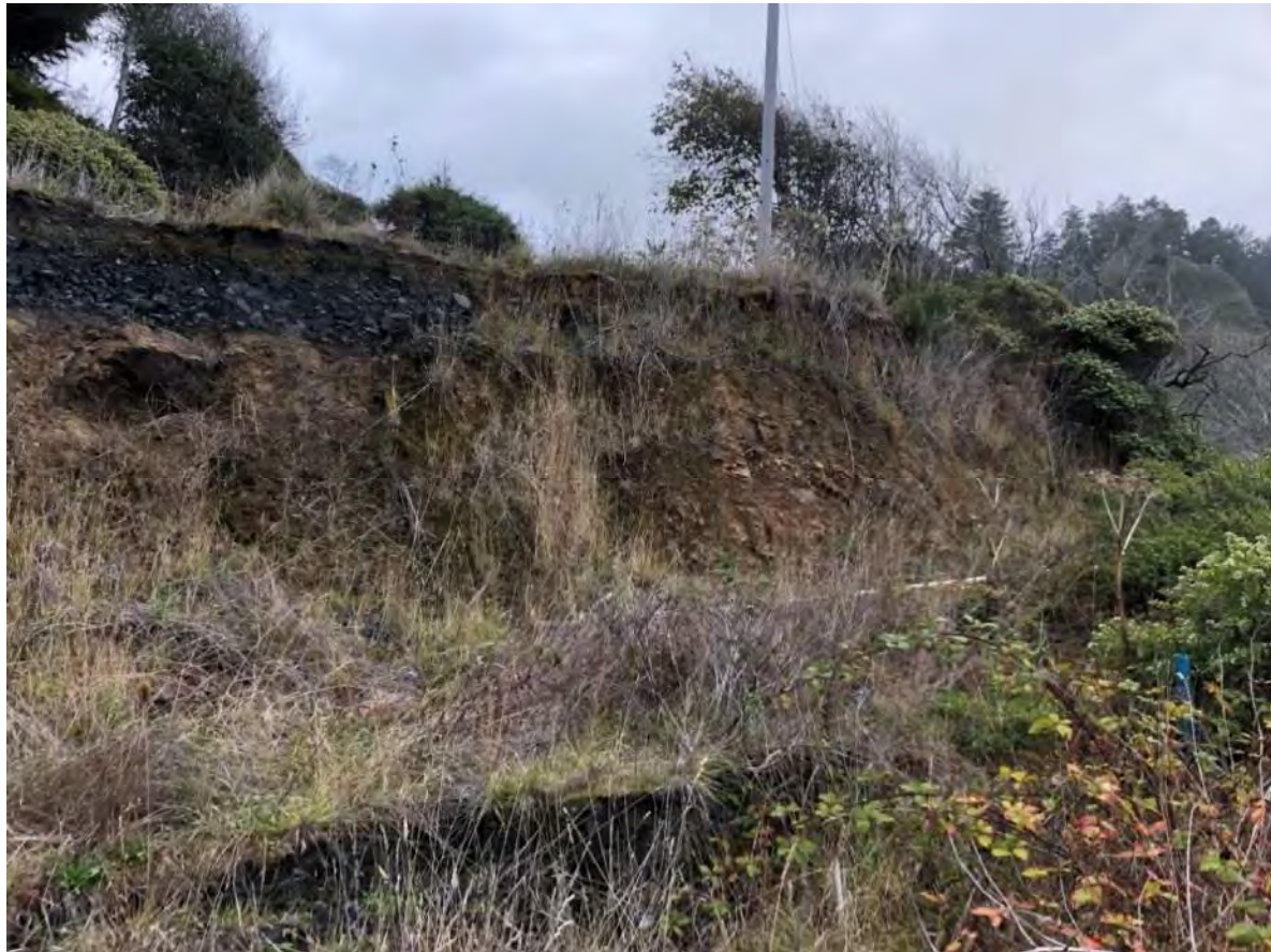
Exhibit 13: Slope failure cutting access road in the southwestern portion of the slide downslope of US 101.
