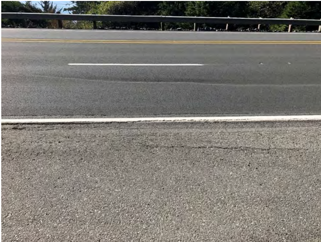
Exhibit 18: Paved over head scarp within US 101 northbound travel lanes.
