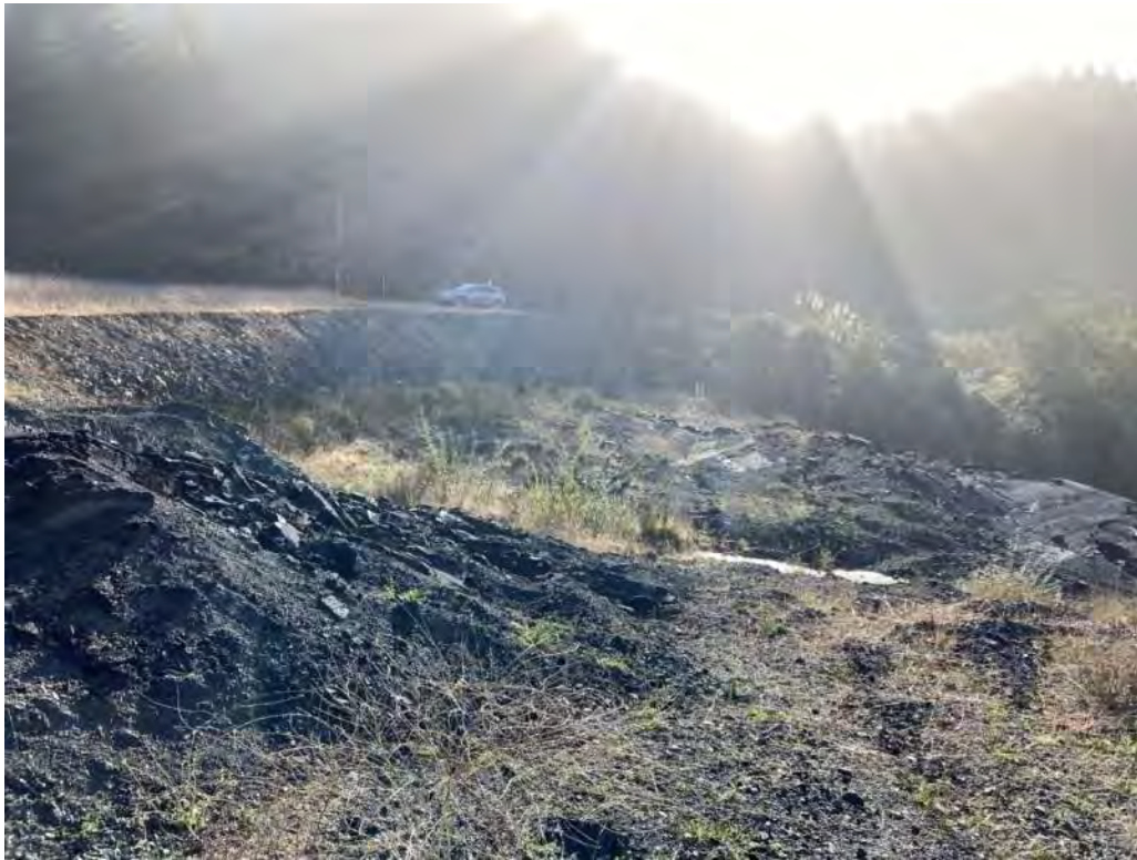
Exhibit 24: Large sections of pavement and road debris below US 101 southbound
