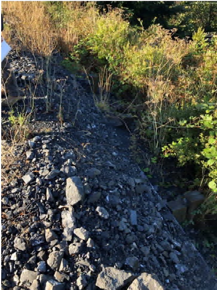
Exhibit 4: Old guardrail with several feet of vertical offset along US 101 southbound.
