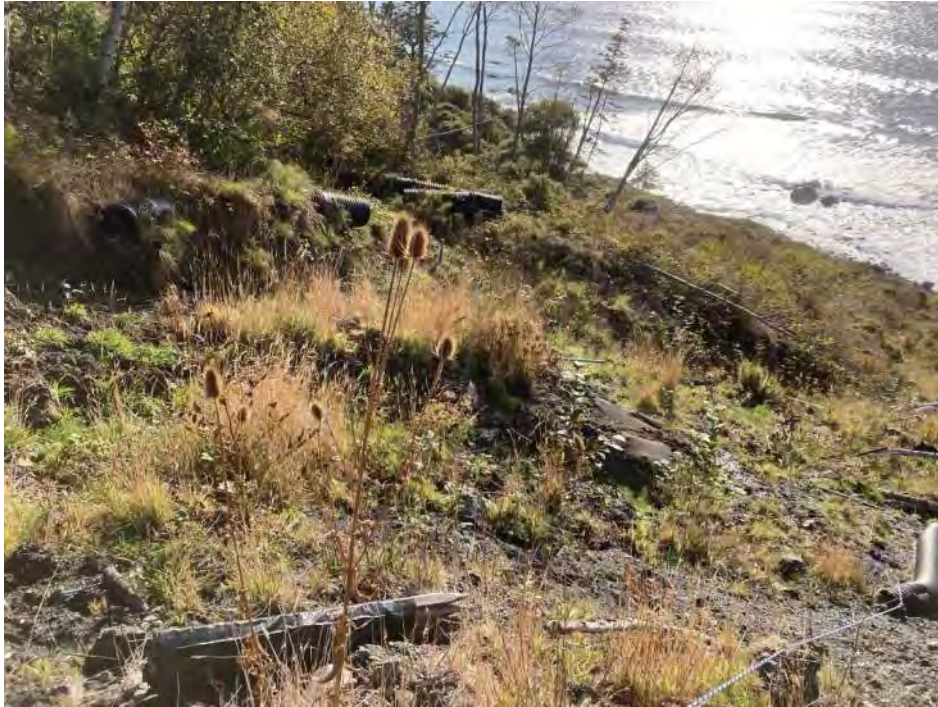
Exhibit 10: Recent secondary slope failure below US 101 that has damaged existing drainage pipes.
