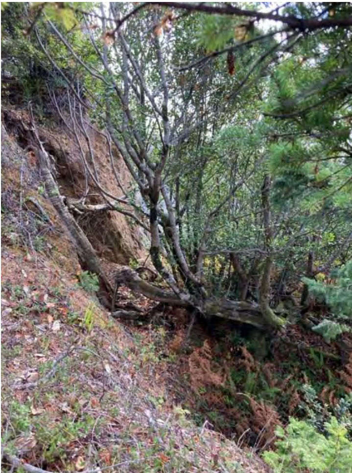
Exhibit 7: Active scarp on the cliff facing the coastline (on back side of cut along US 101 southbound).
