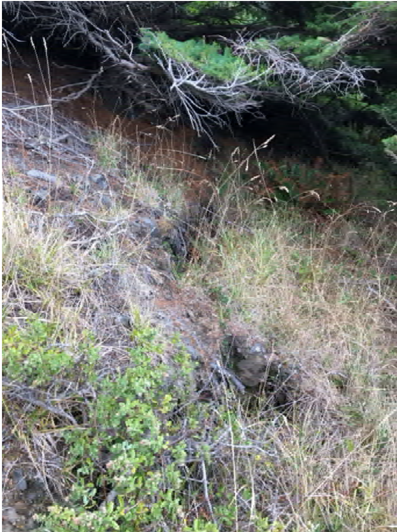
Exhibit 6: Tension cracking located approximately 20 to 30 feet upslope from the top of the rock buttress.
