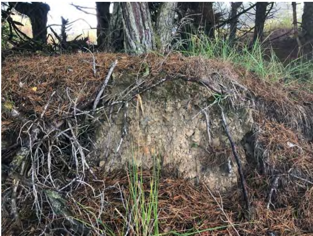
Exhibit 2: Recent scarp movement observed downslope from US 101.
