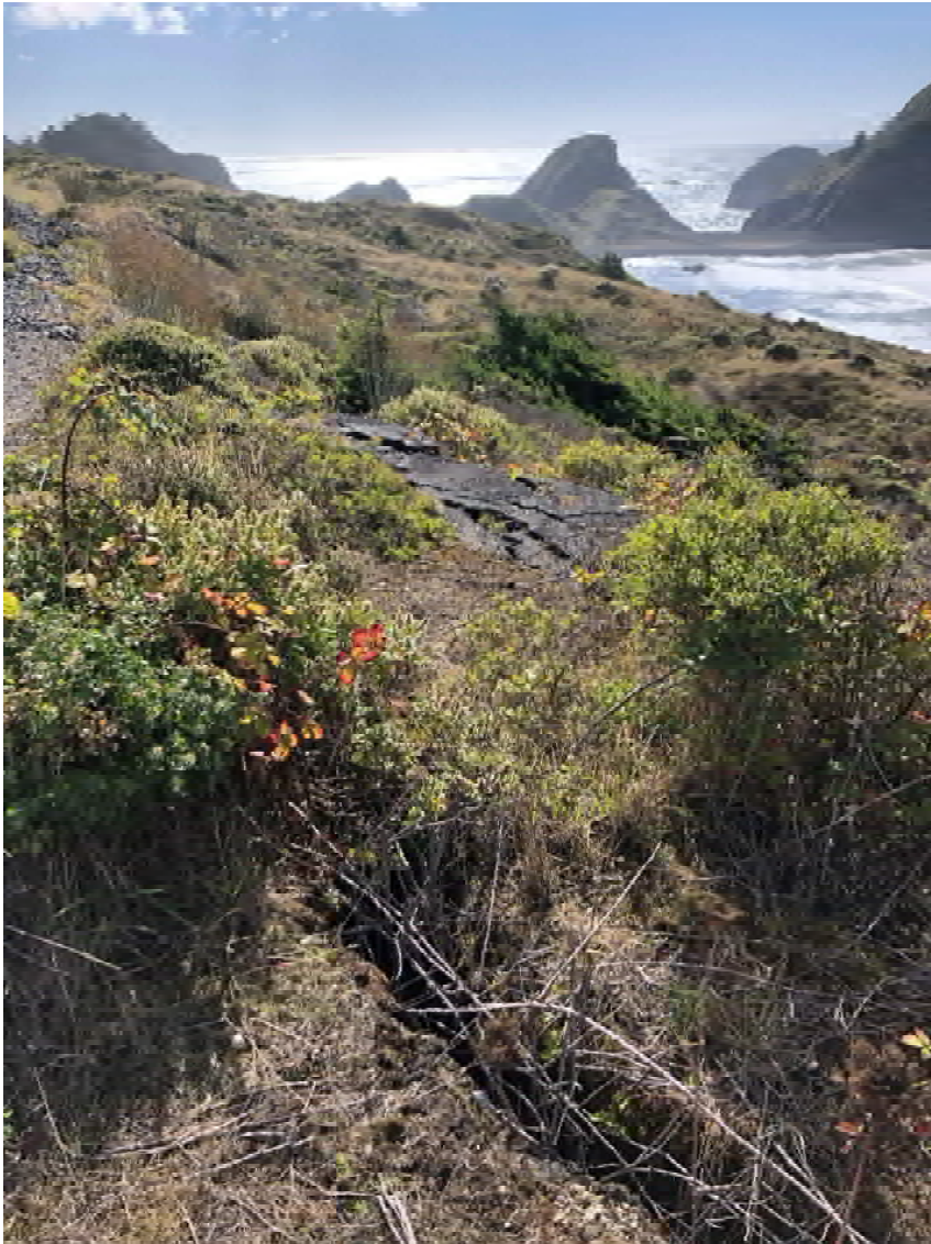
Exhibit 15: Large sections of asphalt with tension cracking downslope of US 101 southbound, potentially the old highway.
