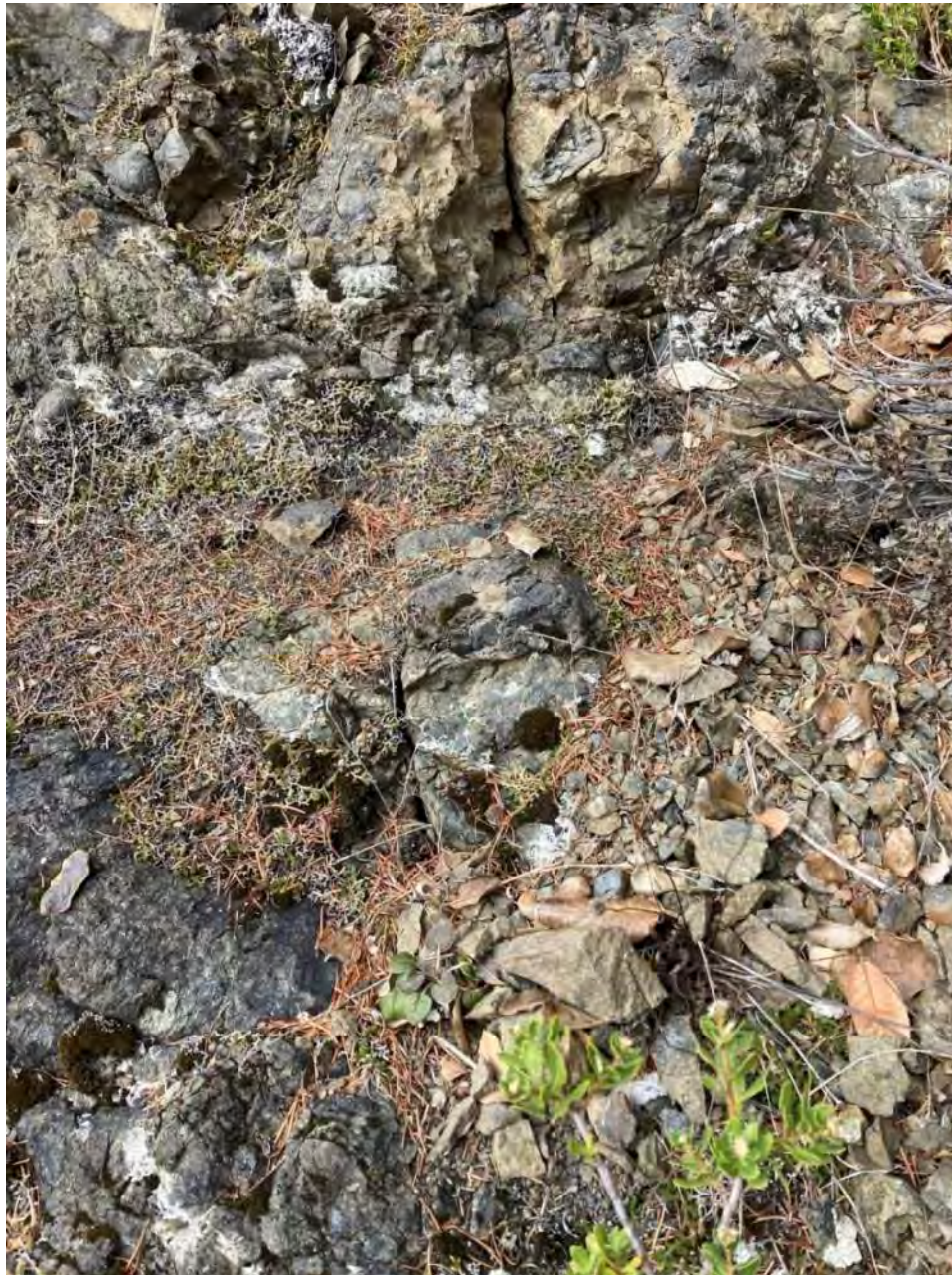
Exhibit 8: Tension cracking in rock outcrops on cliff facing the coastline.
