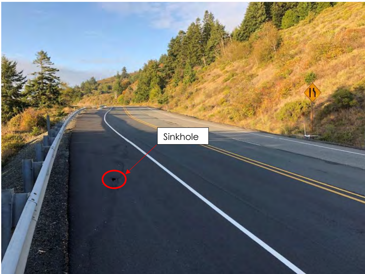
Exhibit 11: Cracking and sinkhole along US 101 southbound indicative of head scarp.
