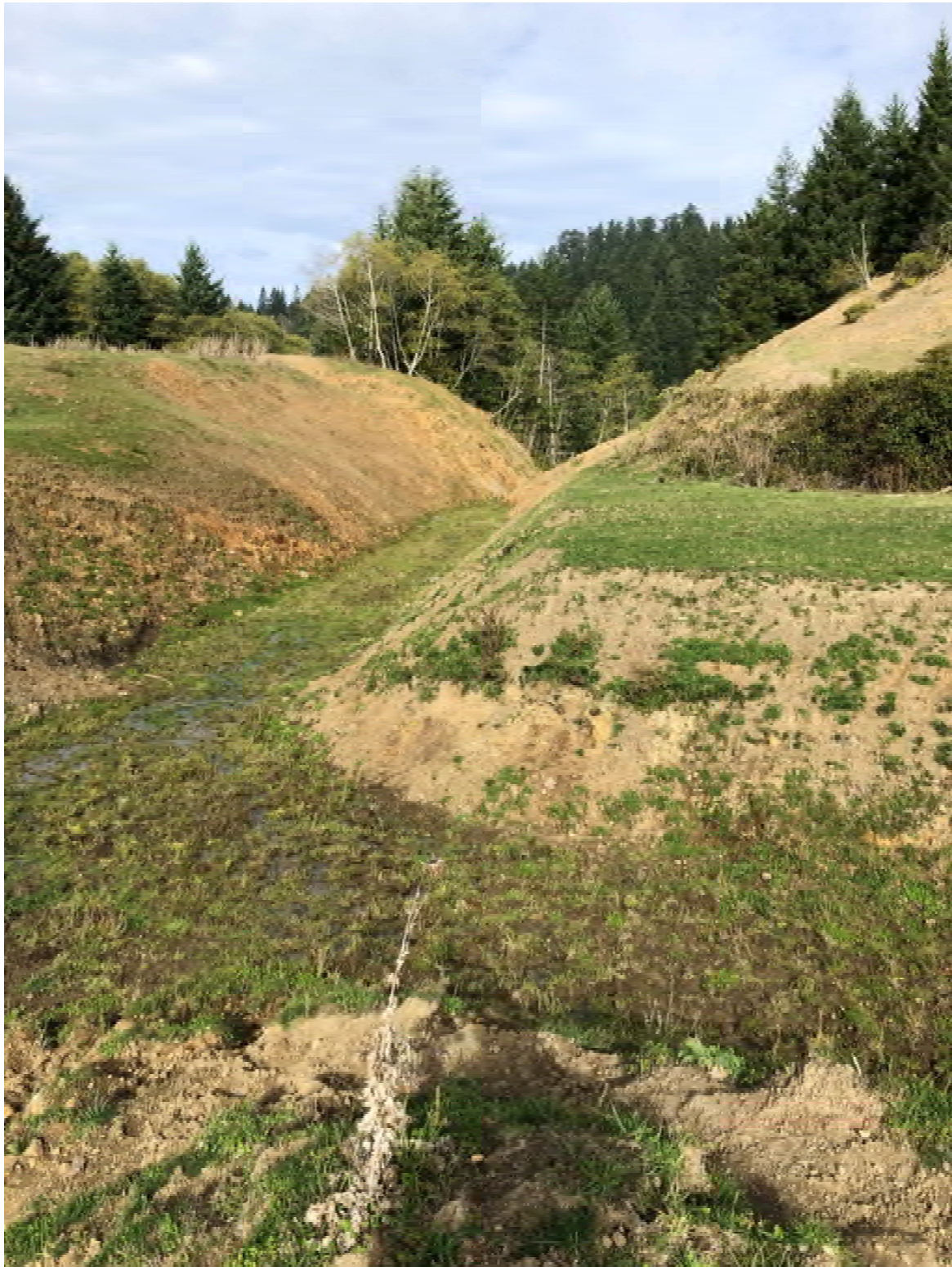
Exhibit 23: Drainage channels within the upper head of the slide constructed by ODOT
