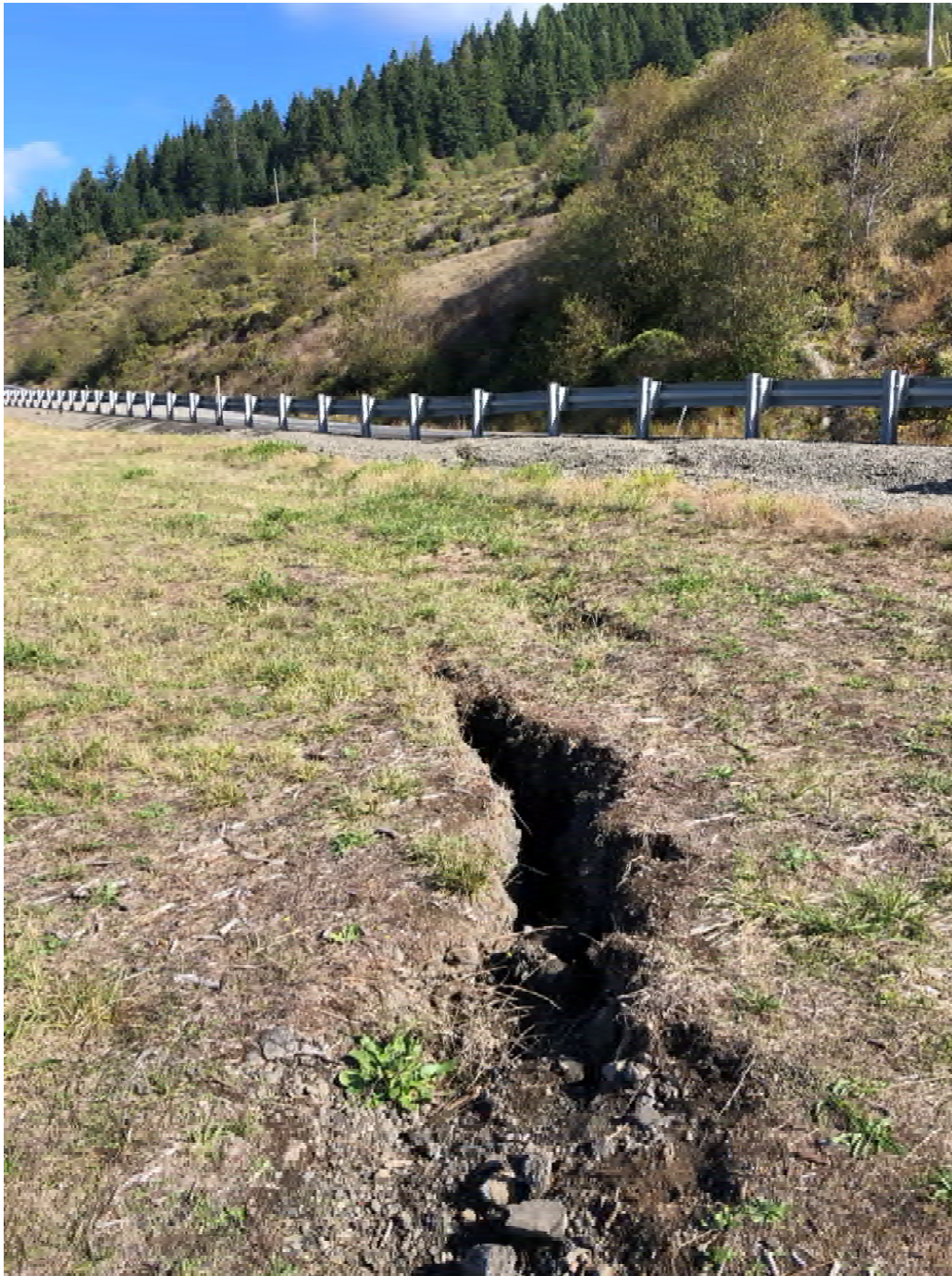
Exhibit 12: Large tension crack at the southern margin of the active slide area, along US 101 southbound shoulder.
