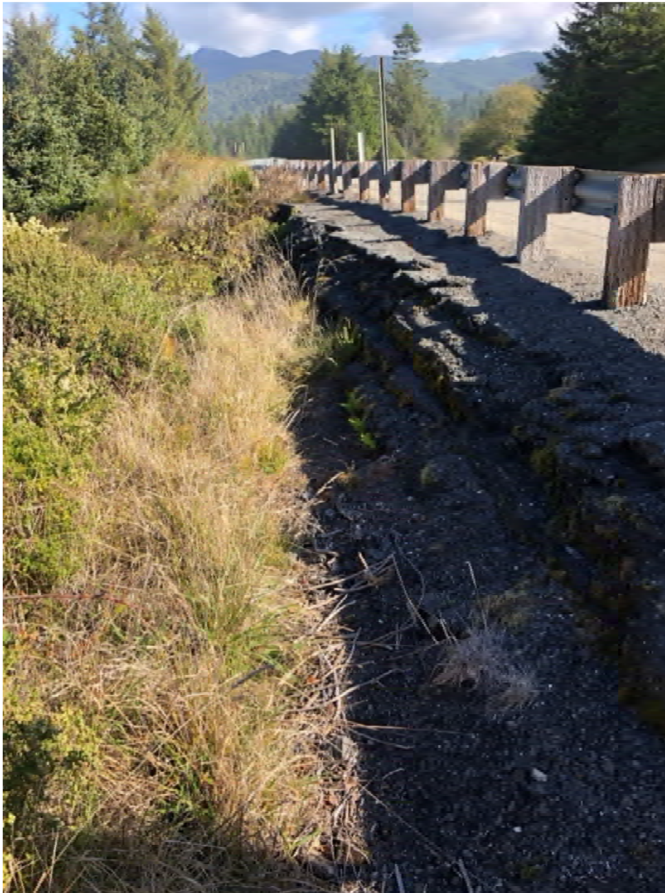
Exhibit 14: Multiple layers of asphalt pavement on US 101 southbound shoulder indicating ongoing displacements.
