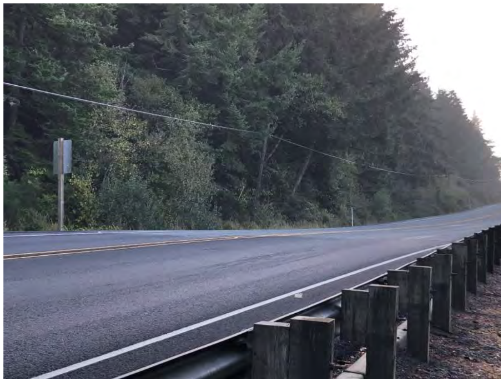
Exhibit 22: Leaning power pole and pistol butted trees just upslope of US 101 northbound
