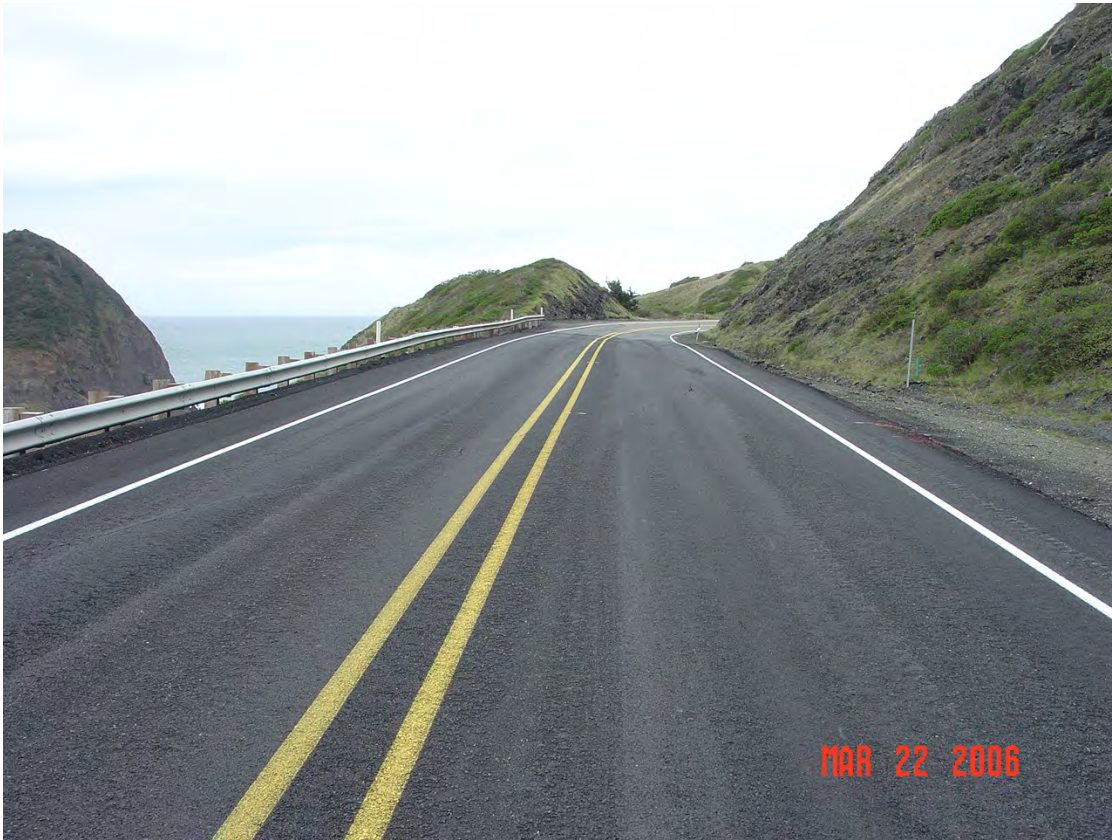
Exhibit 1: Photo looking north along US101, displaying pavement distress within the Frankport South slide limits. Photo taken March 22, 2006.
