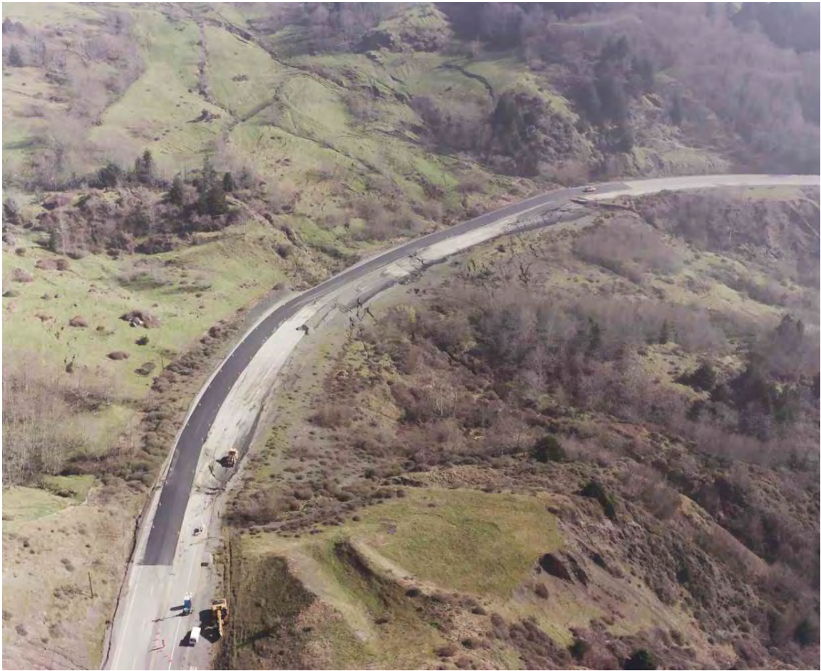
Exhibit 1: Aerial photo looking south at US101 within Hooskanaden Slide limits. Photo taken February 10, 2006
