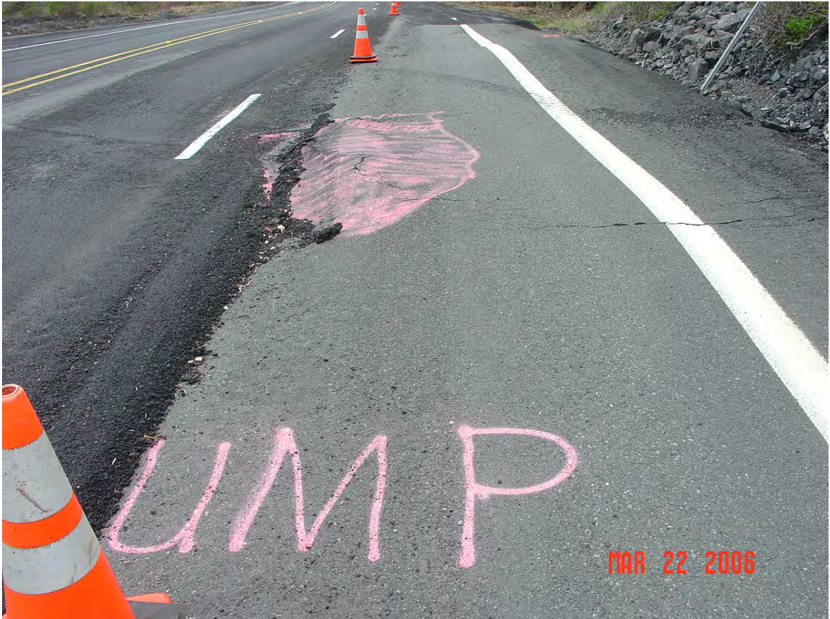
Exhibit 1: Photo looking north at pavement distress within the North Brush Creek Slide limits. Photo taken March 22, 2006.
