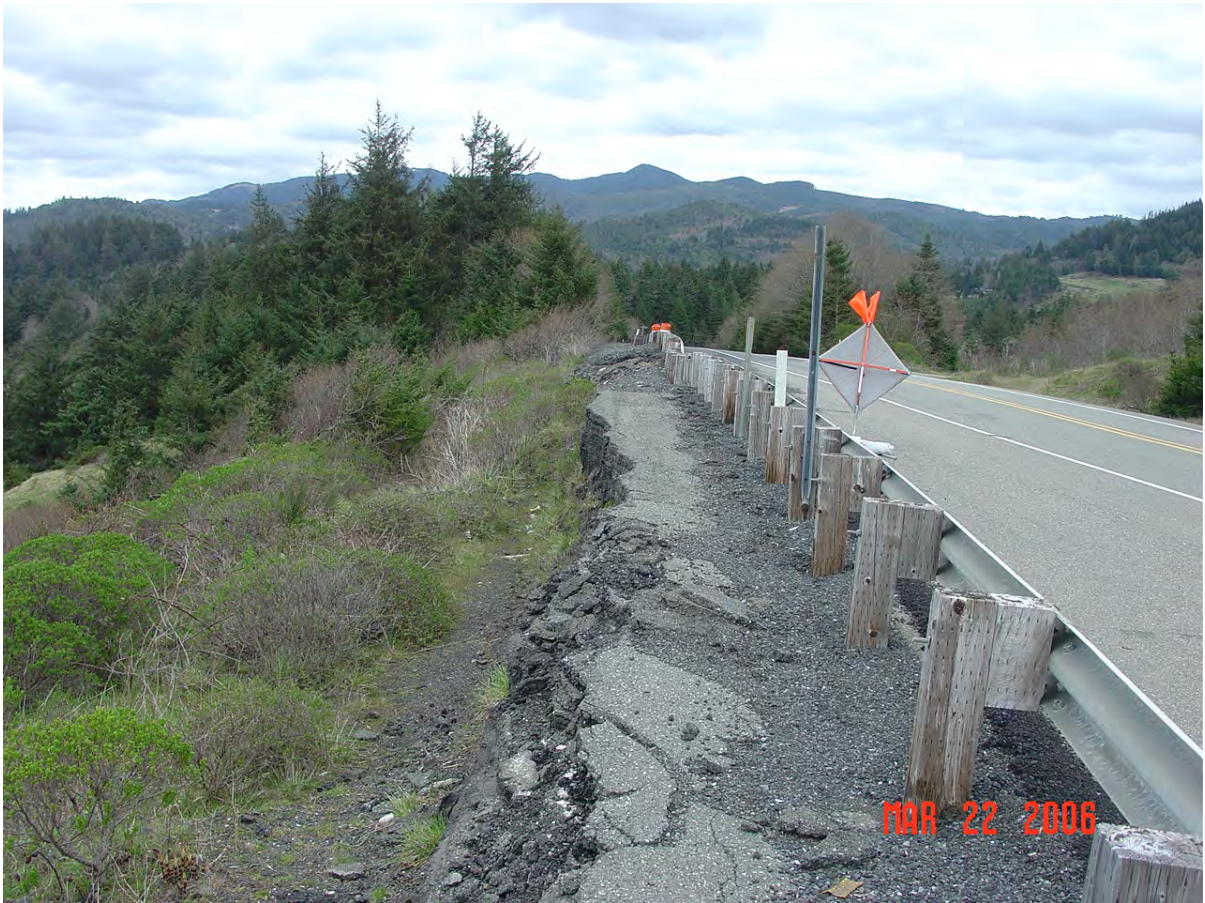
Exhibit 1: Photo looking northeast at the head scarp of the Frankport North slide. Photo taken March 22, 2006.
