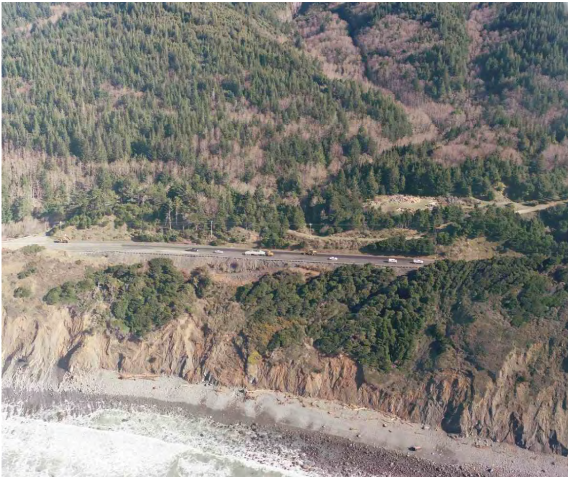
Exhibit 1: Aerial photo looking east at US101 within the Retz Creek South slide limits. The photo shows recent repavement of US 101. Photo taken February 10, 2006.
