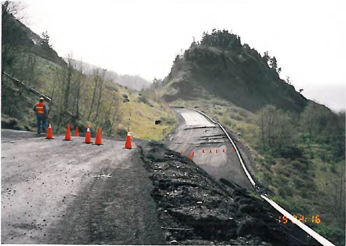
Exhibit 1: Photo looking south along US101 after the 1993 slide event.
