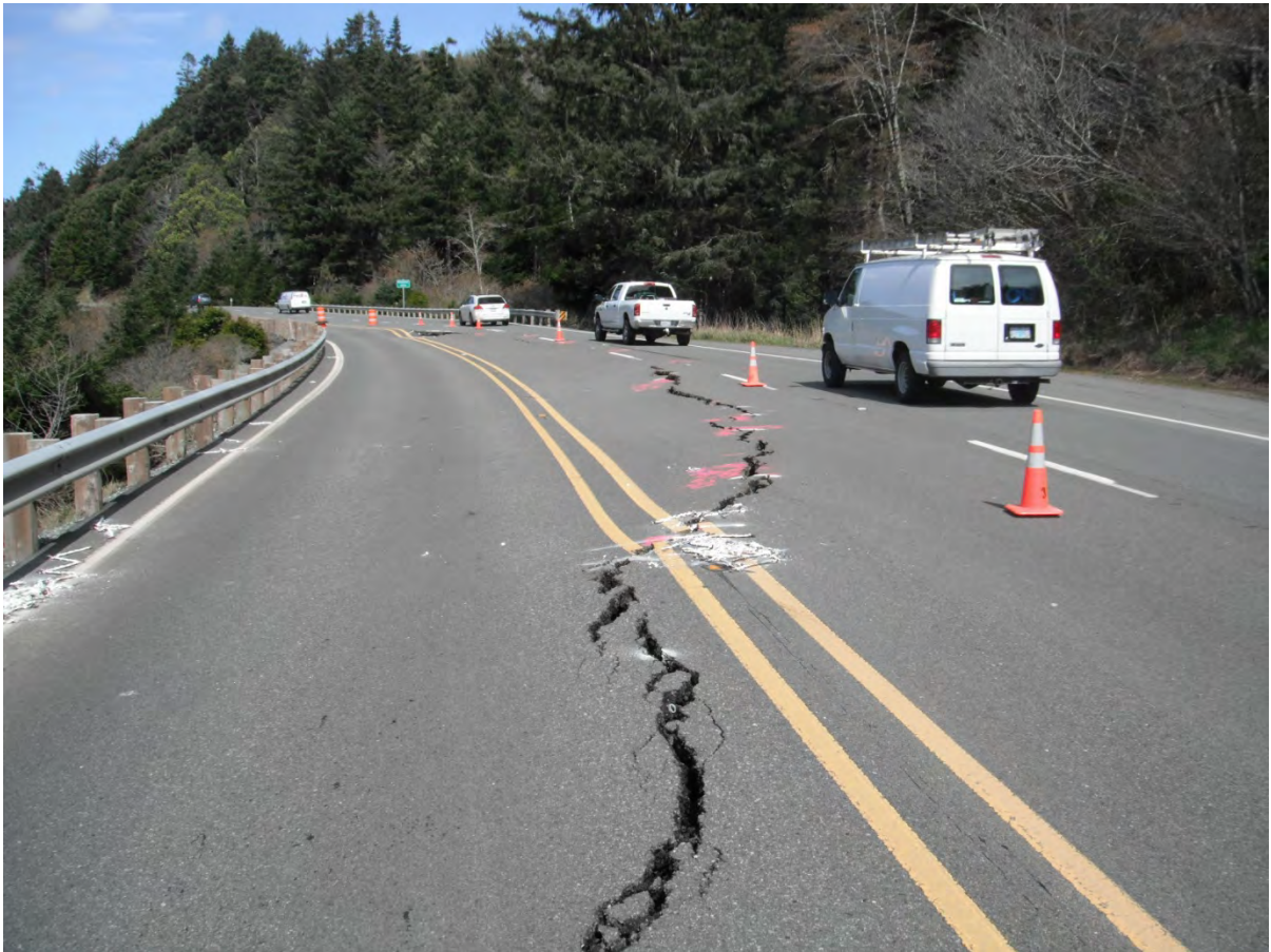
Exhibit 1: Photo looking north along US101 at the Woodroof Creek head scarp. Photo taken March 23, 2012.
