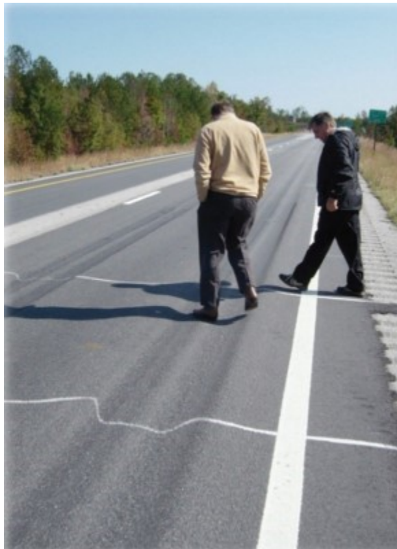
Figure 2.6. Rutting in the pavement due to high binder content and low air void in the asphalt mix (McDaniel and Levenberg 2013)
