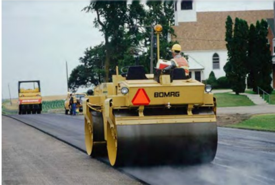
Figure 2.20. Compaction of unsupported free edge by steel wheel roller (Benson and Scherocman, 2006)
