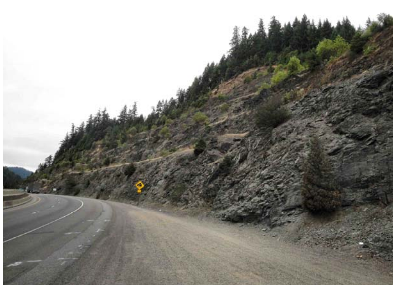
Figure 4.23: View of the Stage Road Pass Summit from I-5's northbound lane. In the highwall of the roadcut, the rock is metatuff
