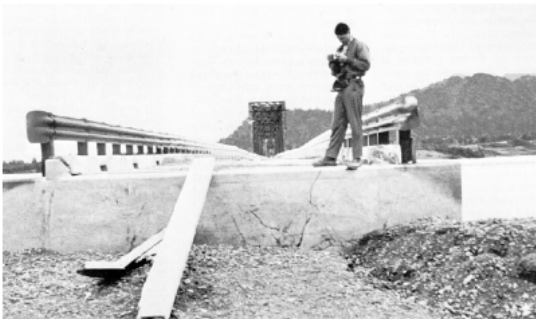
Figure 2.10(b): Post-earthquake Settlement at Copper River Bridge 334
