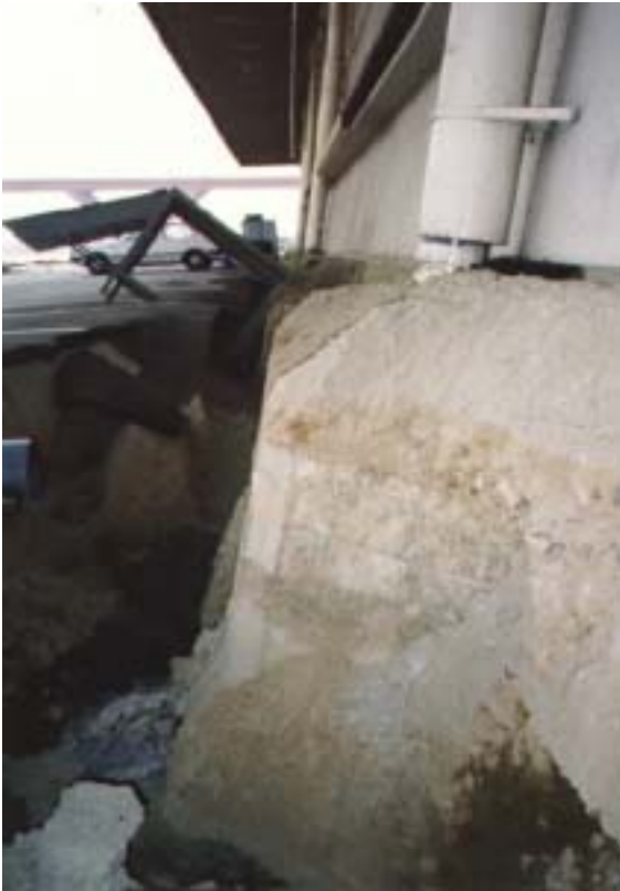
Figure 2.36: Damage to Structures near the Nadahama Ohashi Bridge
