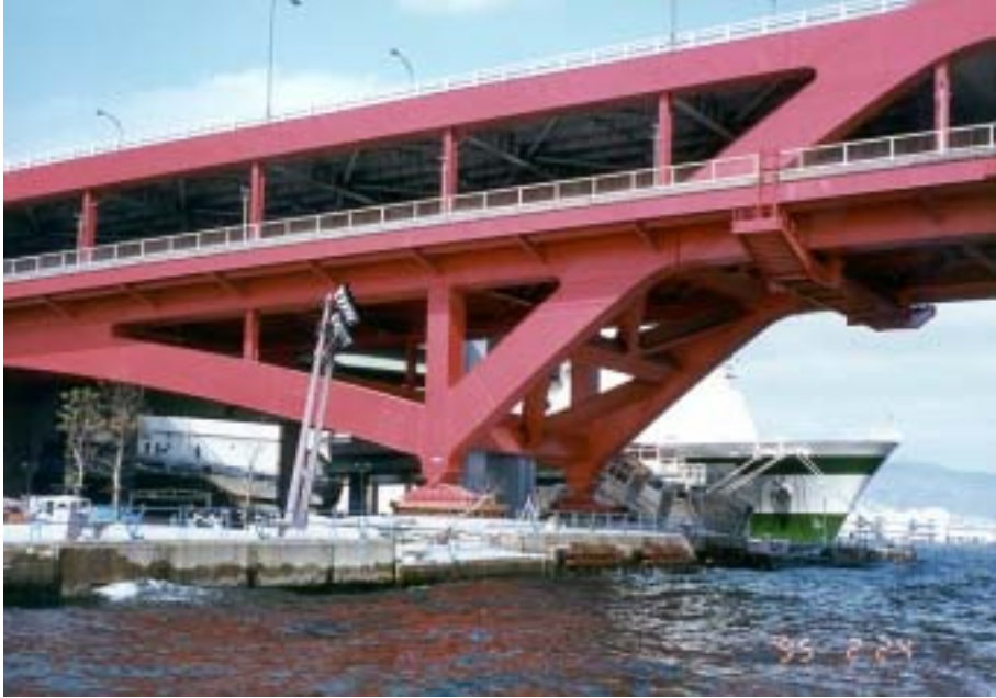
Figure 2.32: Kobe Ohashi Bridge Damage
