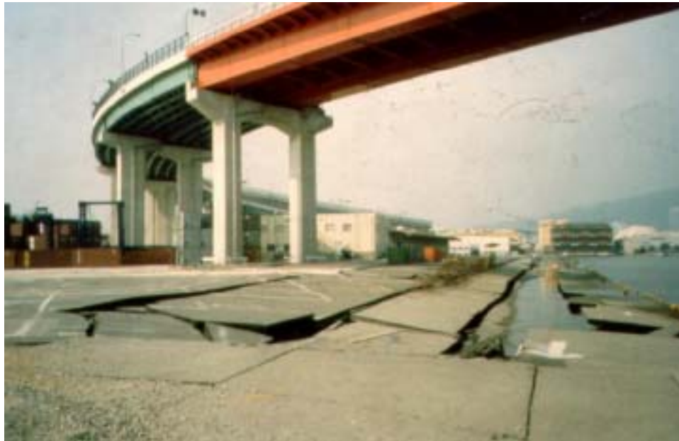
Figure 2.34: Nadahama Ohashi Bridge Lateral Spreading of 3 to 4 m
