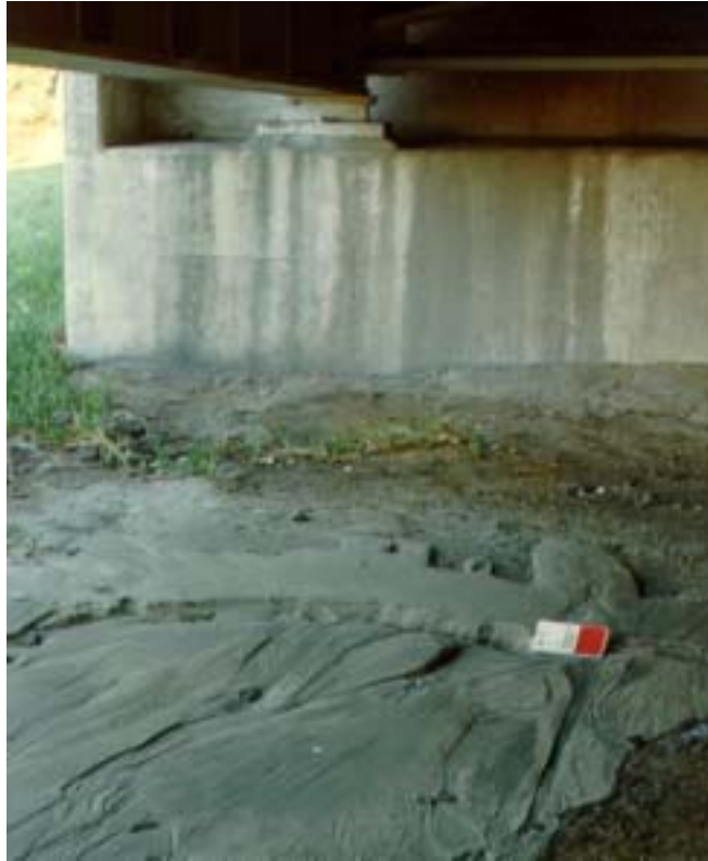
Figure 2.24: Sand Boils at the Oakland-San Francisco Bay Bridge Approach Fill
