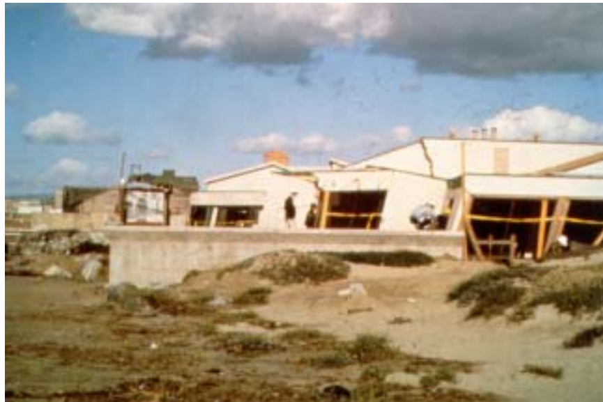
Figure 2.18: Damage to the Moss Landing Research Facility due to Settlement and Lateral Spreading
