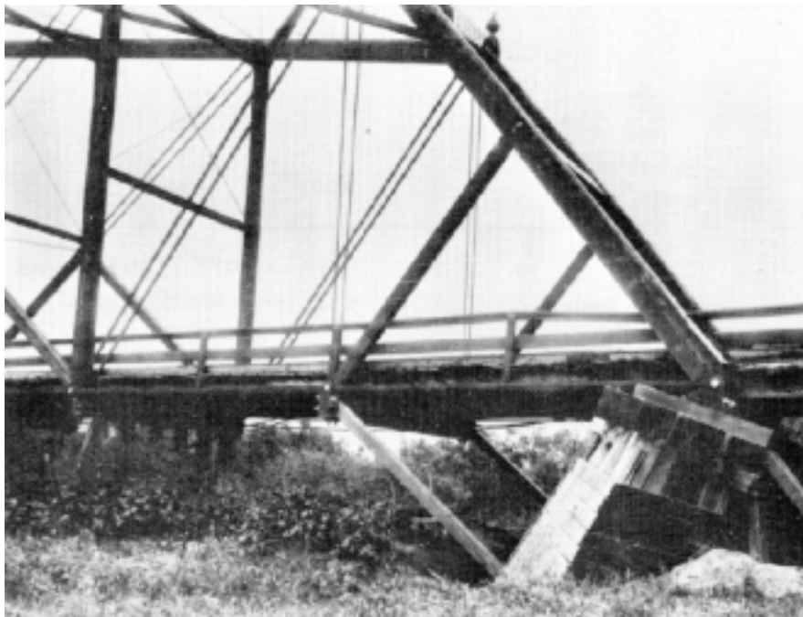
Figure 2.20: South Terminal Pier of Bridge over Salinas River 6.4 km South of Salinas
