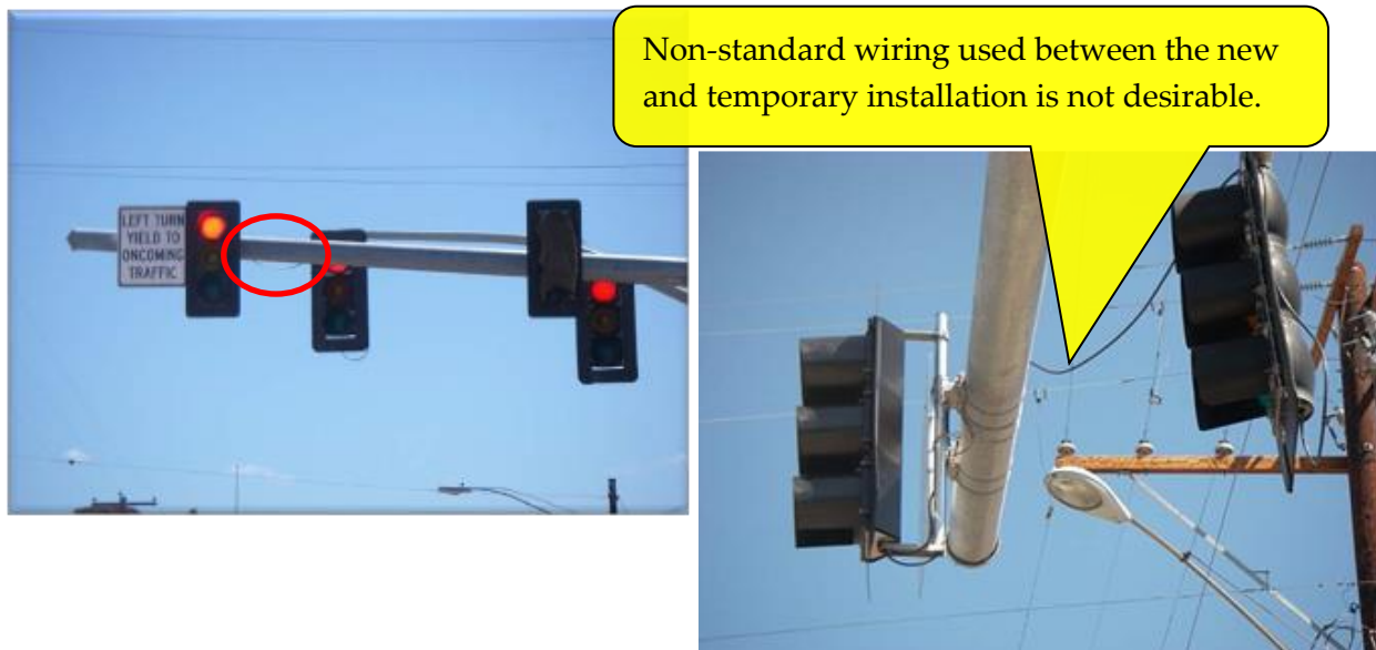
Figure 11-5 | Use of New Equipment for a Temporary Installation – This Practice Not Allowed
