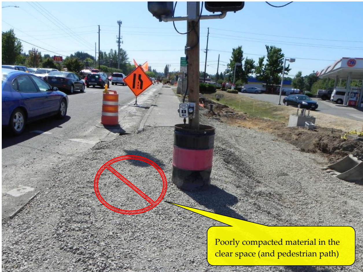
Figure 5-71 | Poorly Compacted Material Example
