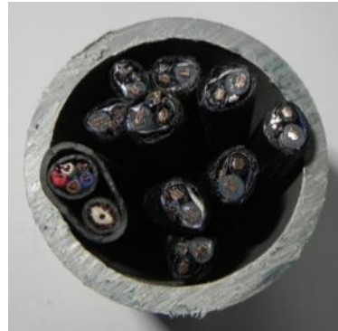
1 1/2" conduit w/9 loop feeder cables + 1 video cable Exceeds NEC max fill Exceeds ODOT max fill
