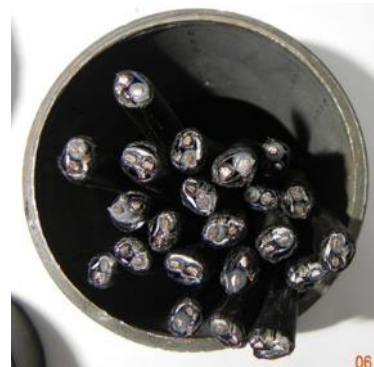
3" conduit w/22 loop feeder cables Does NOT exceed NEC max fill Does NOT exceed ODOT max fill
