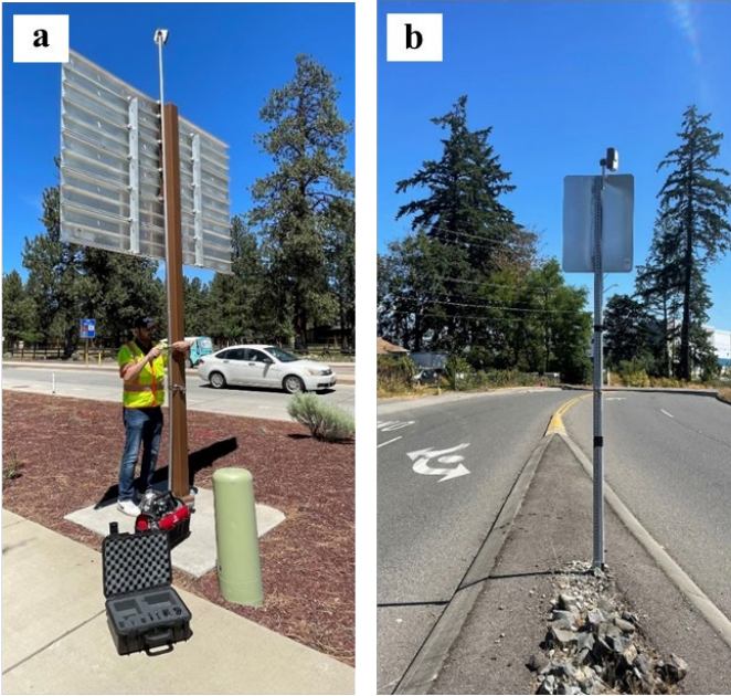
Figure 3: Equipment Installation on (a) Southbound Approach in Sisters, OR and (b) Camera in Field on Westbound Approach in Lakewood, WA
