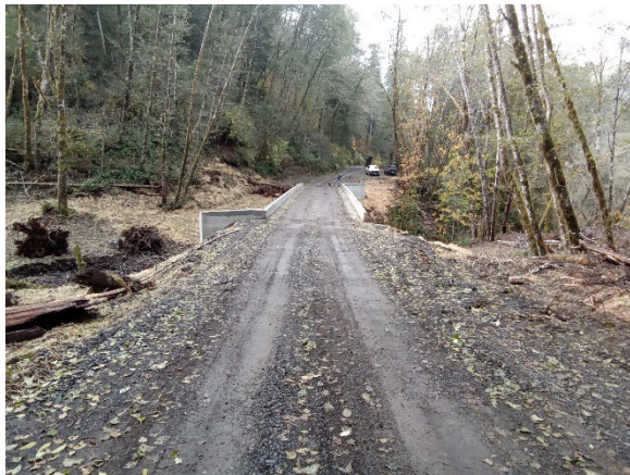
Bridge replacement in the Tillamook State Forest. Stream crossing improvements can help protect water quality, reduce the risk of flood damage, and improve aquatic habitat by enabling organism passage to upstream habitats.
