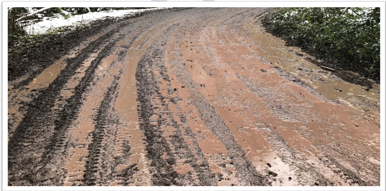
Photo 5. Road surface with a layer of mud and rutting [recommend using a different image].
