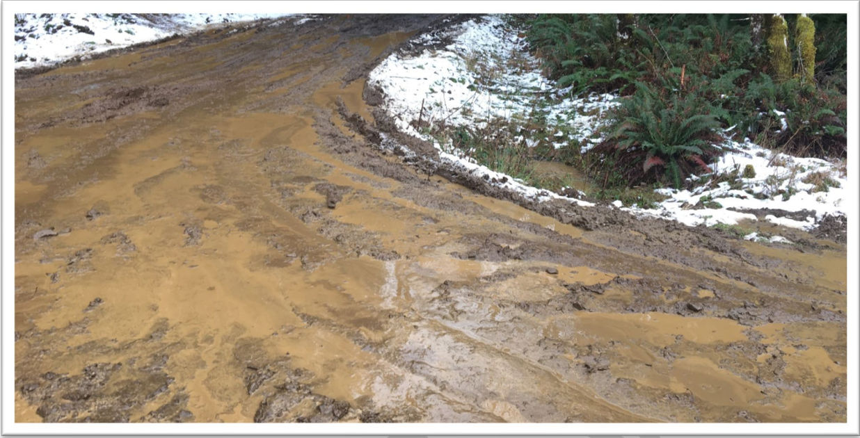
Photo 5. Road surface with a layer of mud.
