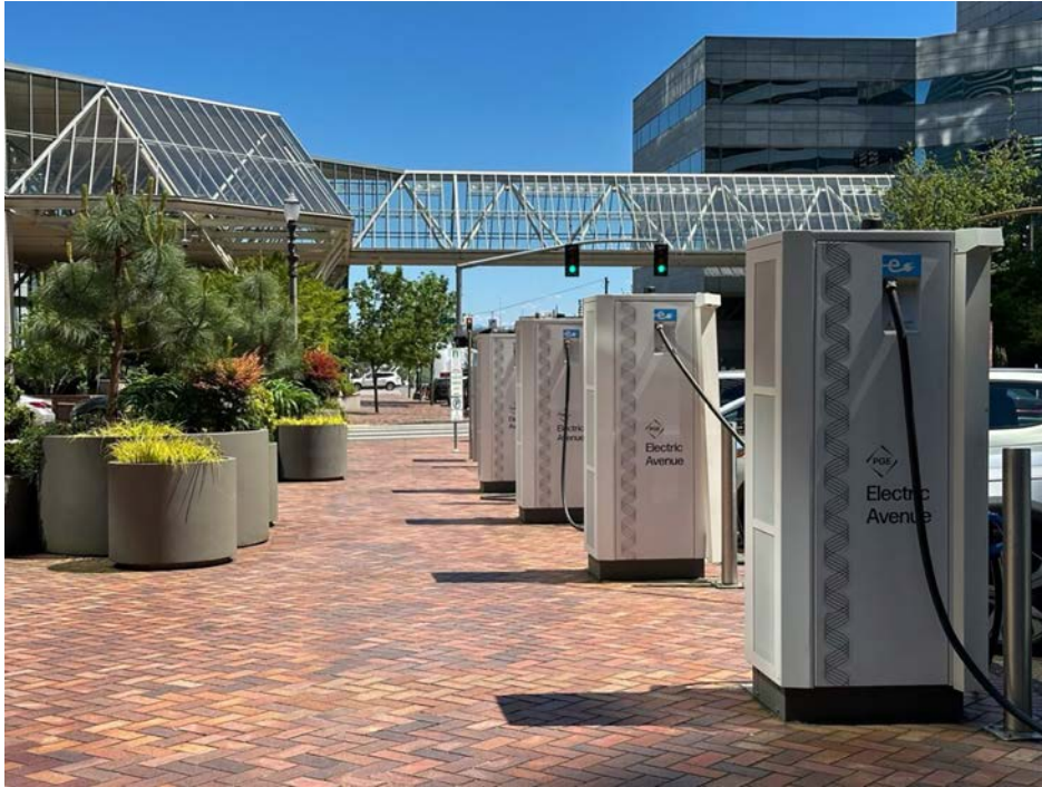
Figure 7: “Electric Avenue” along SW Salmon Street in Portland, one of several on-street sites featuring charging infrastructure installed by PGE
