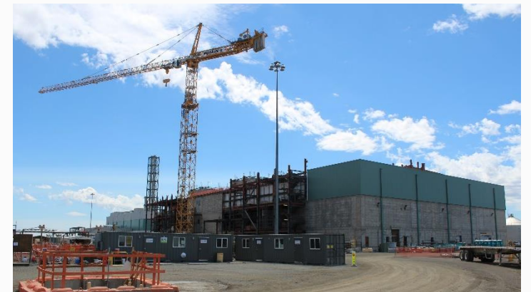
High-level waste facility in 2019. Following increased funding design and construction has recently resumed.
