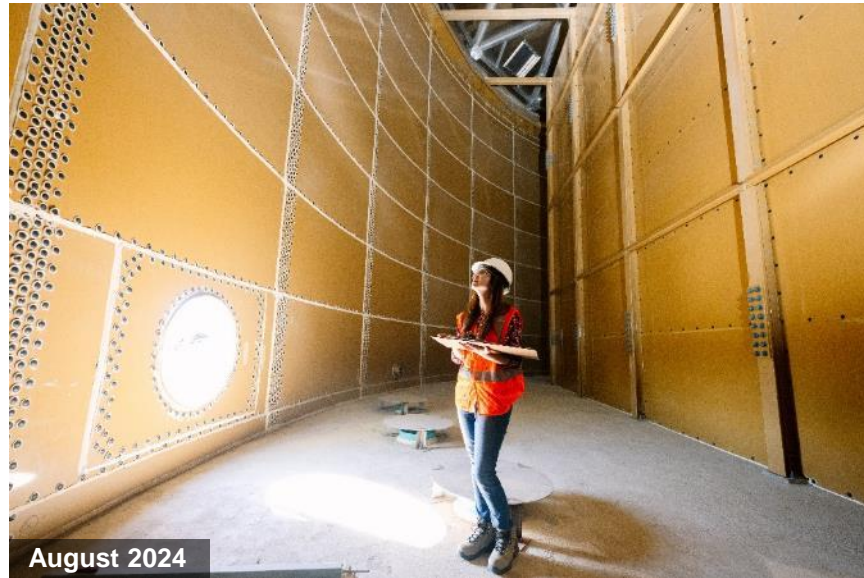
Inside of tank at the Central Plateau Water Treatment Facility
