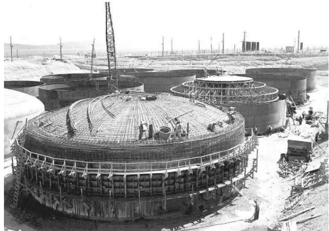
The underground storage tanks under construction. When completed, the top of the tank was covered by 8 feet of soil, and the bottom is about 40 feet below ground.
