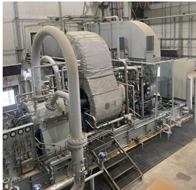
GC500-Installed late 90's
