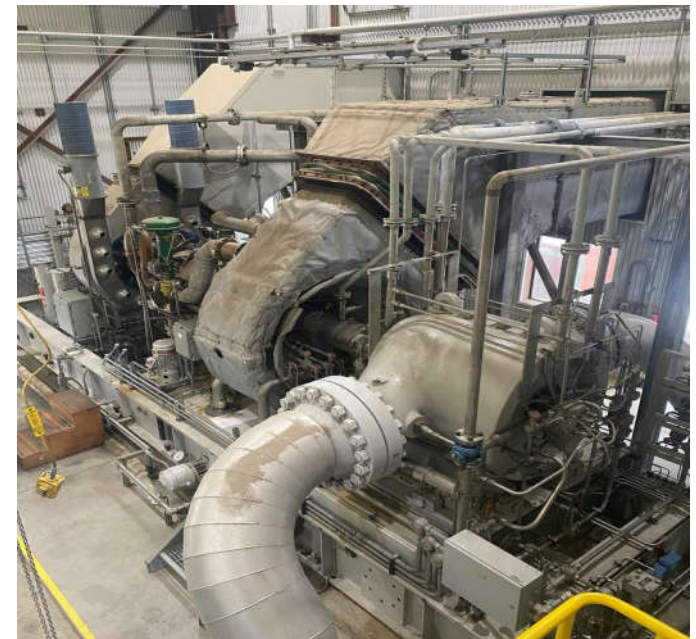
GC600-Installed early 2000's
