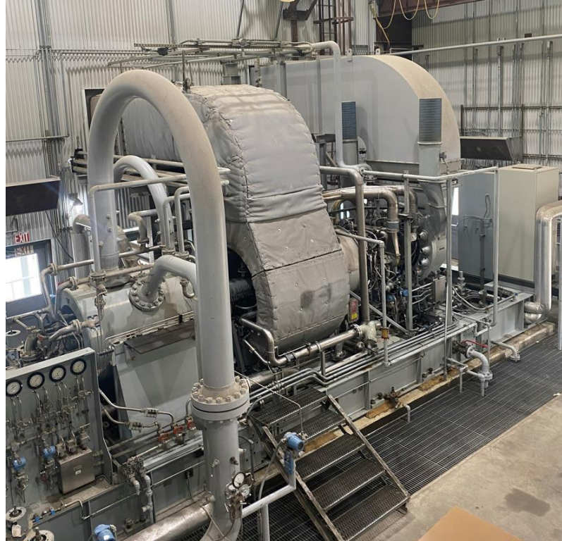
GC500-Installed late 90's
