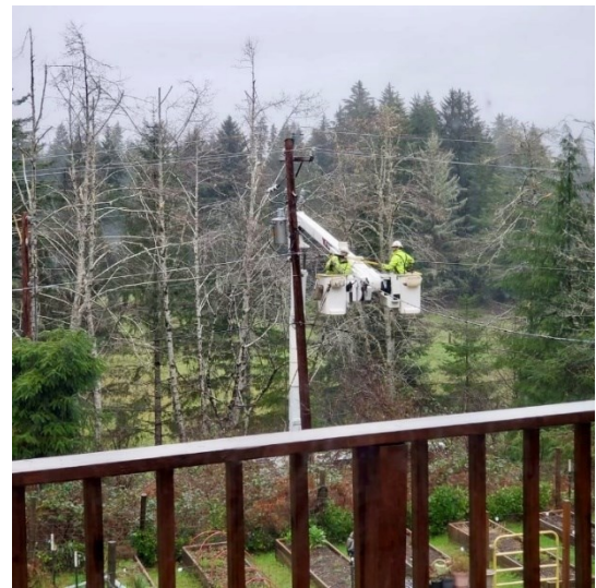
Crews from other electric utilities responded through mutual aid agreements to Central Lincoln PUD’s service area to help repair the system following the January 2024 ice storm.
