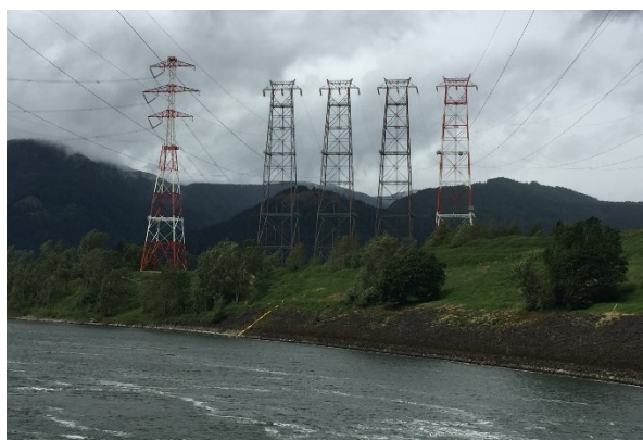
Transmission towers at the Bonneville Dam.
