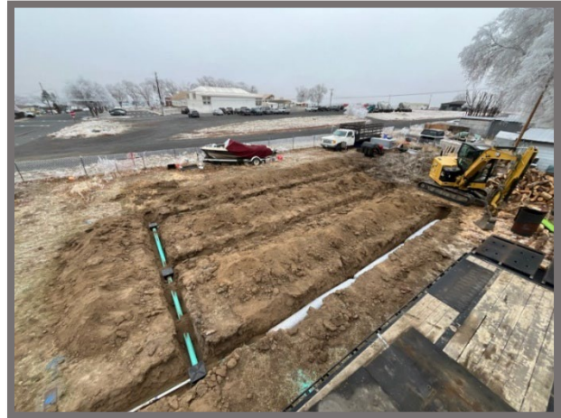
A drain field is installed as part of a major repair in Deschutes County.
