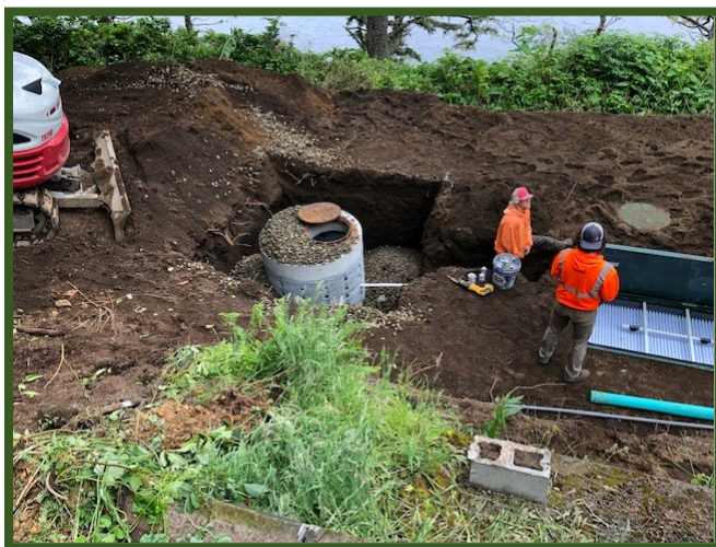
An approved alternate treatment septic system is installed near a waterway in Tillamook County
