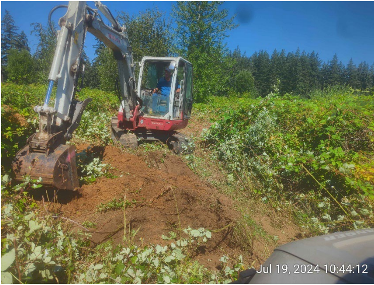
Incremental sampling was done with the assistance of a mini-excavator. Sixty test pits were excavated.
