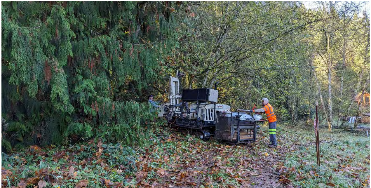
Photo 10. Drilling activities at the westernmost boring location at the Raw Water East assessment location.
