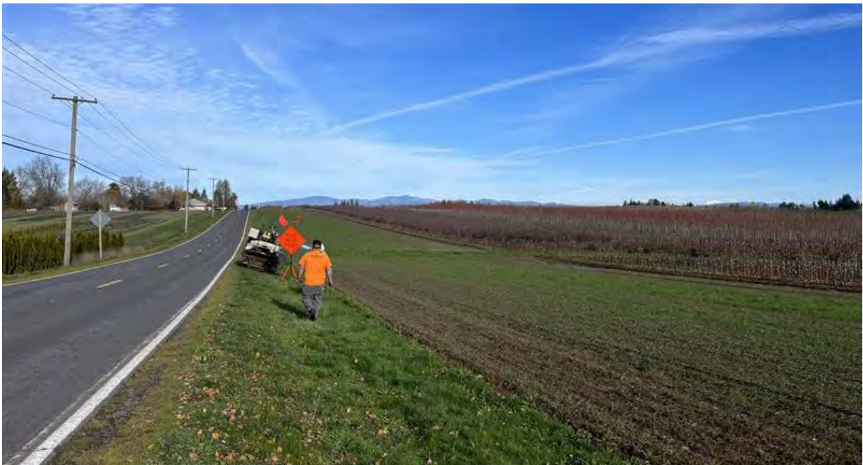
Photo 4. A direct-push drill rig on the shoulder of the SE Altman Road (Finished Water North) assessment location.
