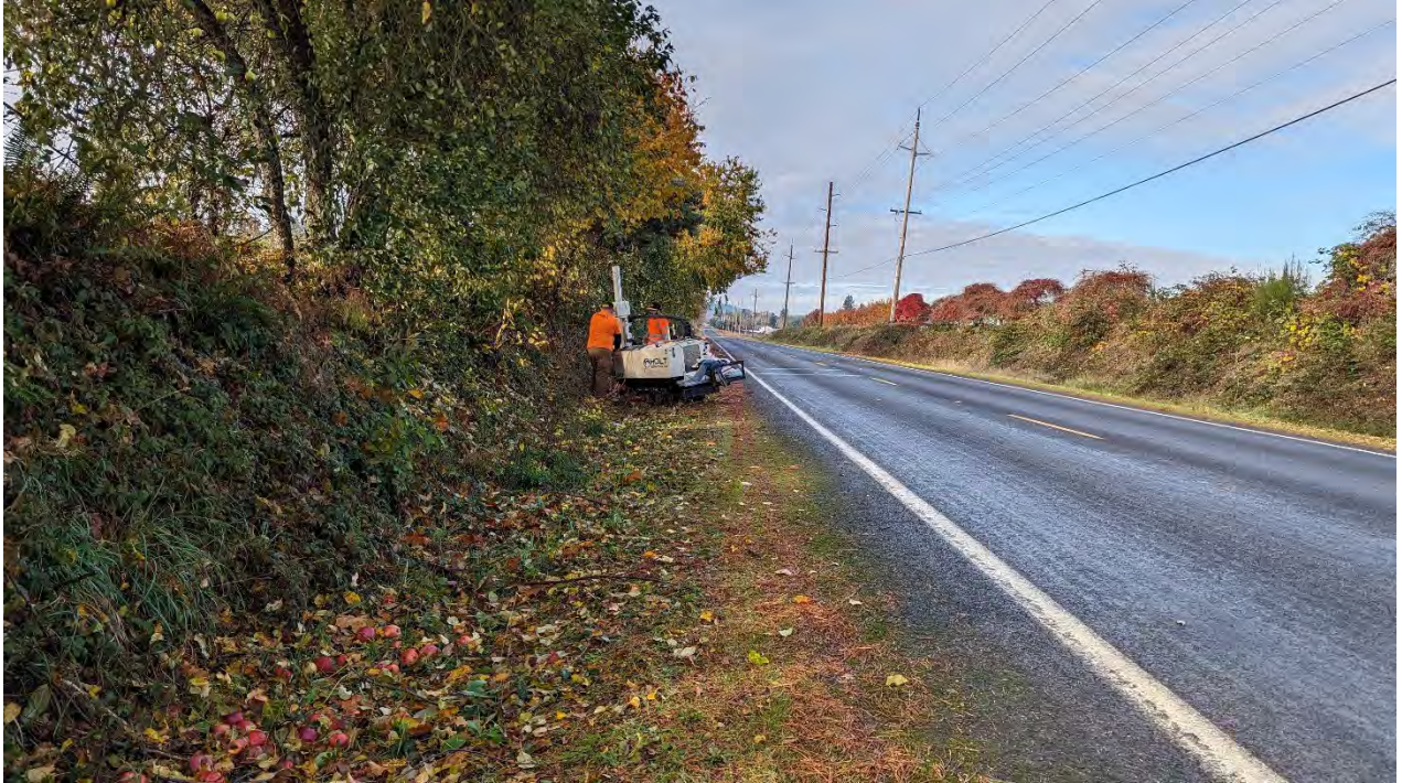
Photo 7. Drilling within the roadway shoulder of SE Dodge Park Boulevard (Finished Water South).
