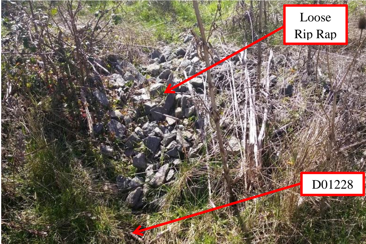
Figure 6: Loose Rip Rap Outfall, looking south
