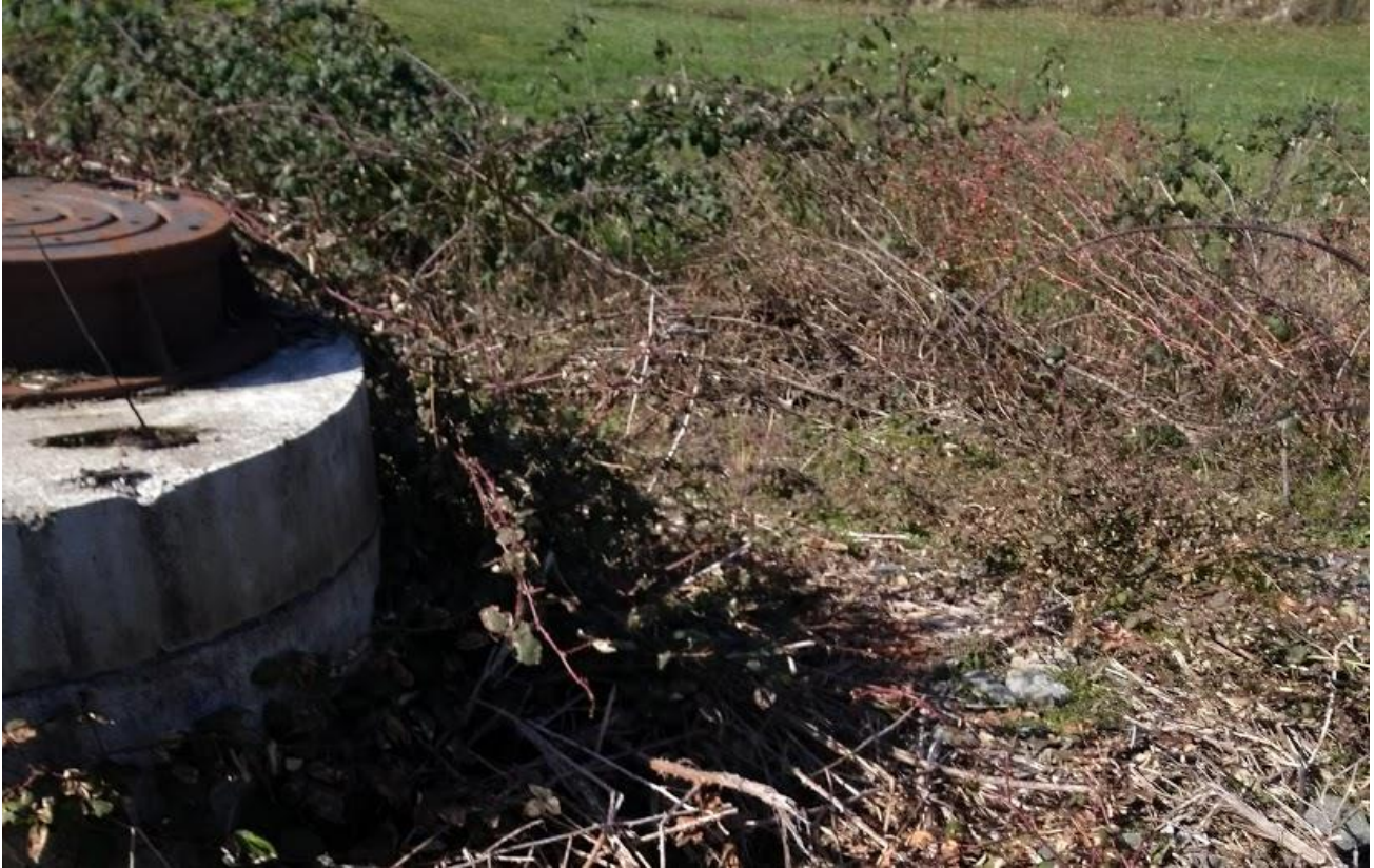
Figure 5: Standard Manhole that leads to water quality facility
