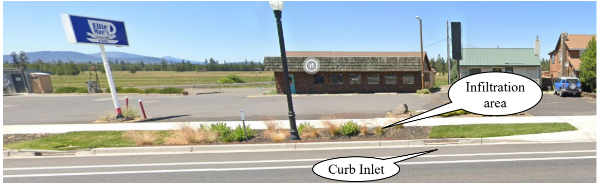
Photo 1: Infiltration area designed to infiltrate a 100 year storm, thus there is no outlet.
