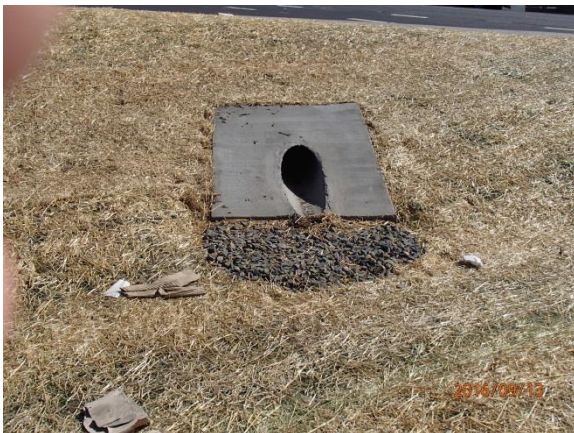
Figure 5: Looking south. Pipe connected to inlet marked as 'A' on operational plan and profile.
