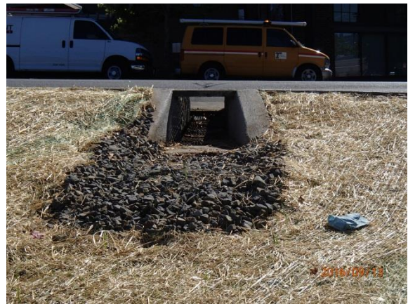
Figure 6: Looking south. Example of channel and grate type inlet marked as 'B' on operational plan and profile. (2 in facility)
