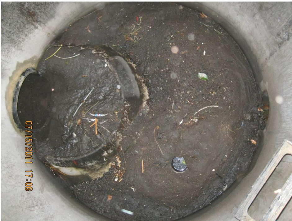
Photo 3: Interior view of Stormceptor water quality manhole, completely silted over and needing maintenance to function properly.
