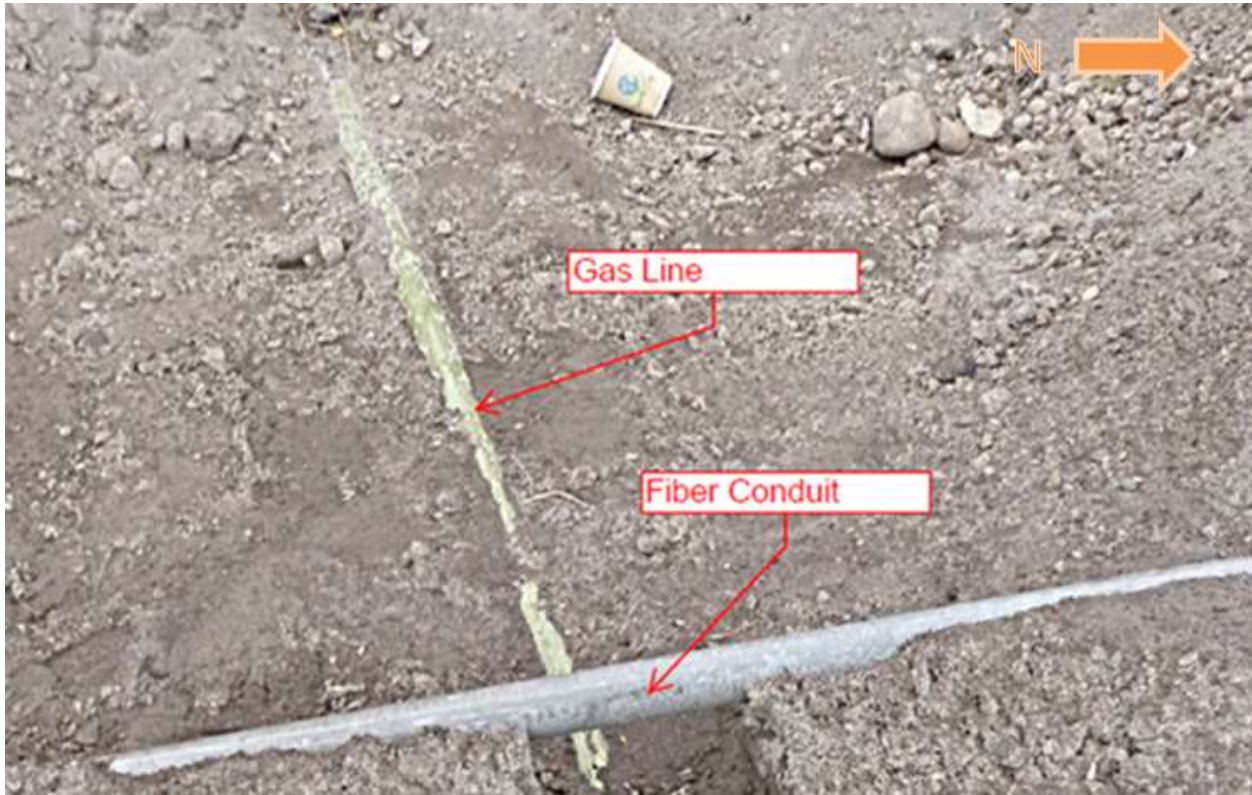
Figure 4: Fiber Optic and Gas conduit running directly under facility. Digging in the facility is NOT ALLOWED.
