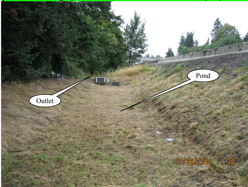
Photo 1: Extended Detention Dry Pond looking north. I-5 is located to the right.
