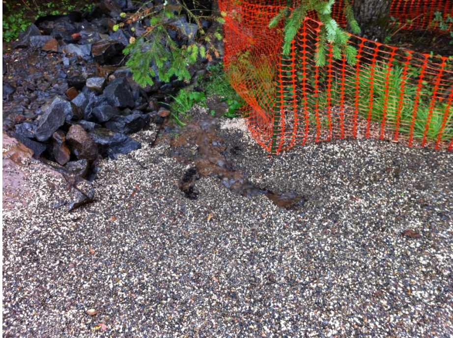
Figure 10: Outlet from both riprap channel and inlet #6 into drainage ditch looking southeast
