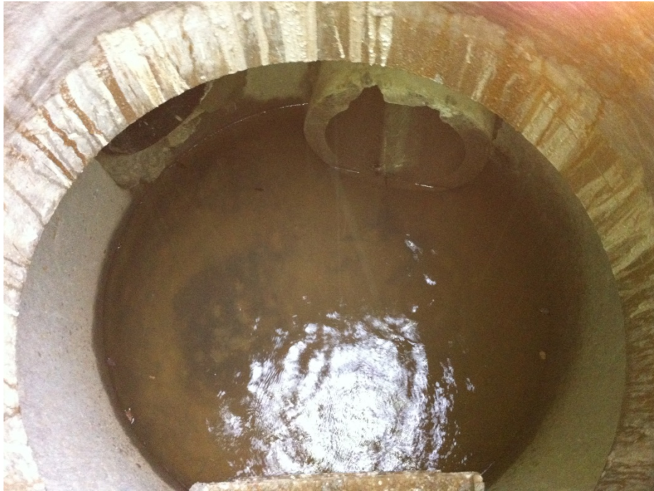
Figure 12: View of storm sewer pollution control manhole
