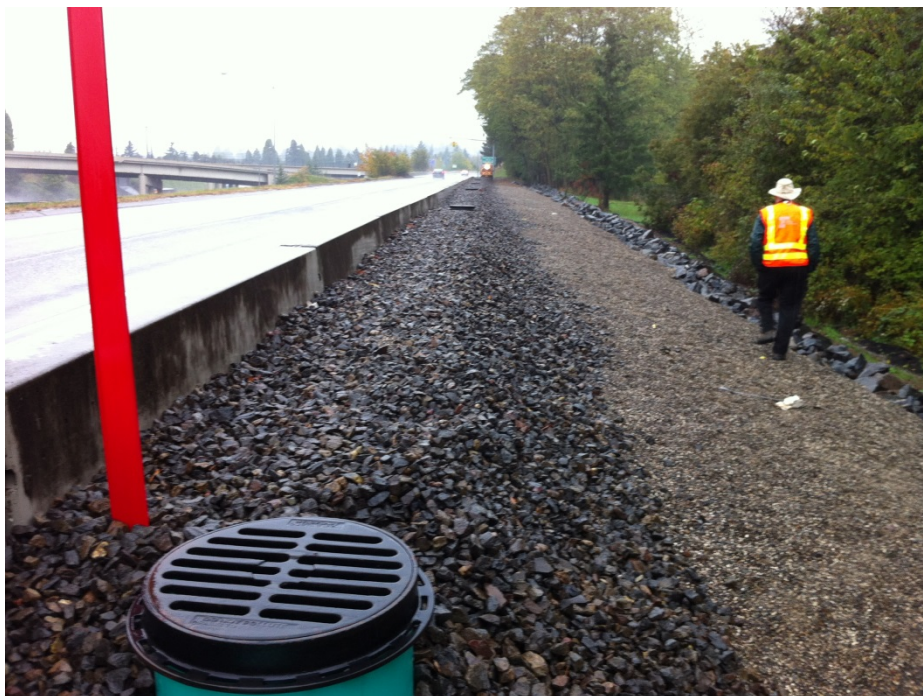
Figure 7: Looking north at bioslope. Southern-most PVC inlet (#6) visible.
