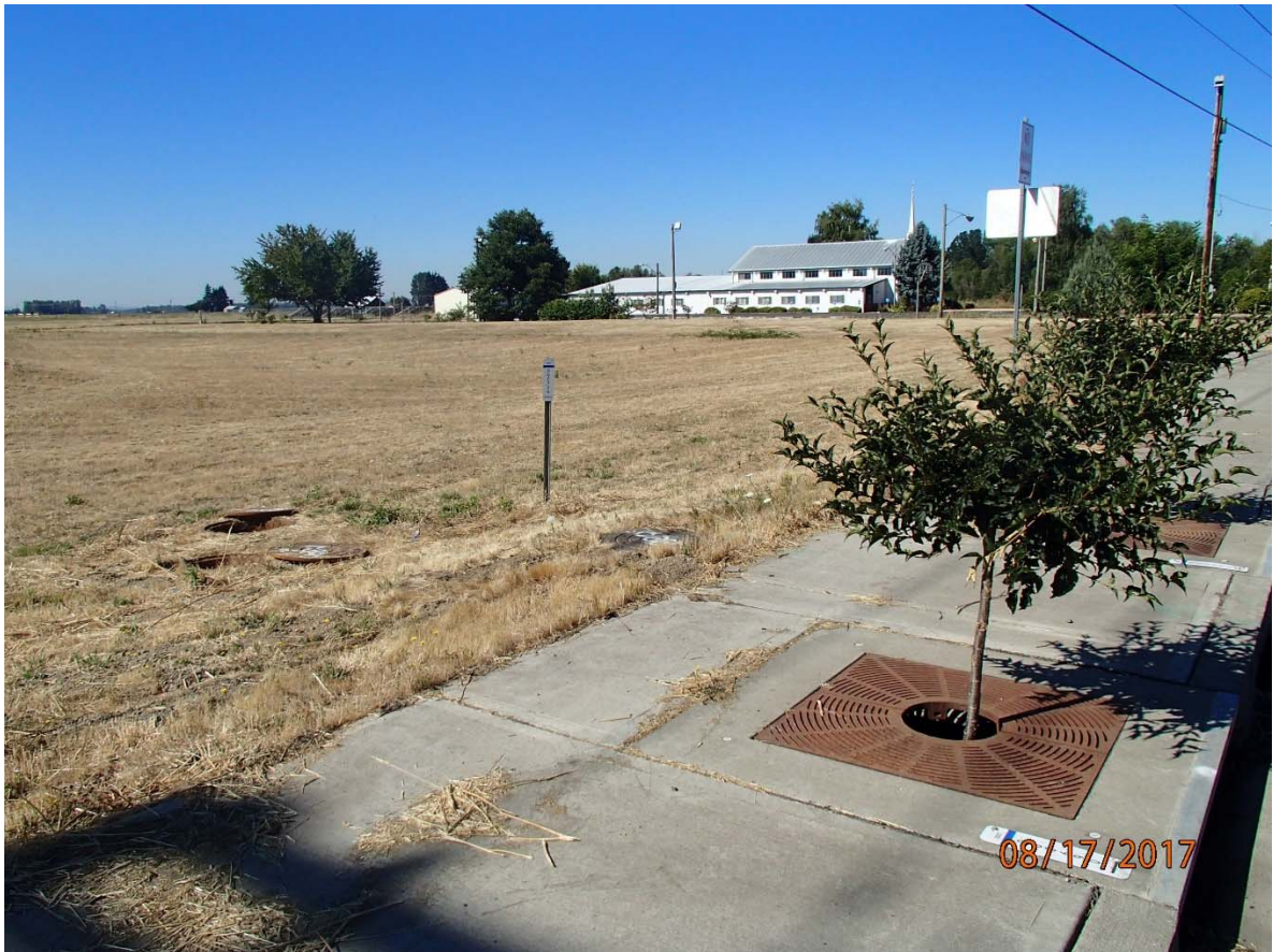
Figure 1: DFI No. D00726, Access to the detention tank flow control manhole at the outlet
