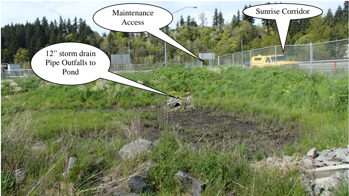
Photo 2: a view of bio- retention pond, looking Northeast toward Sunrise Corridor.
