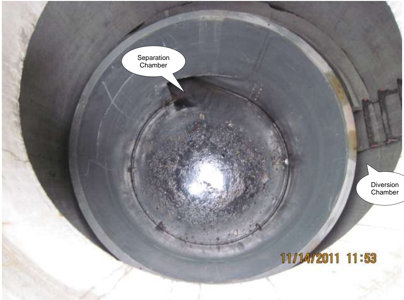
Photo 3: Interior of water quality manhole for this facility D00538.
