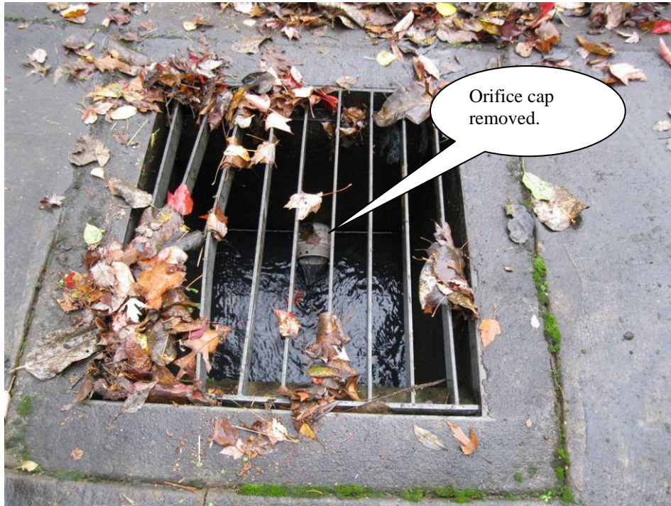
Photo 3: Looking at the secondary inlet/outlet device. Facility was originally designed to contain an orifice cap overtop the pipe exit, above.
