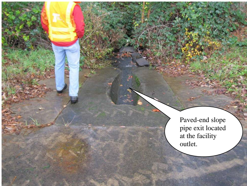
Photo 4: Looking east at the facility outlet, paved-end slope pipe exit and riprap lined outfall to Springbrook Creek – straight ahead.
