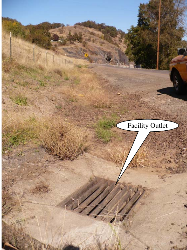
Photo 2: Type G2-MA inlet, considered the facility's outlet control device, is located in the area between McLain Avenue, I-5, and the northbound onramp. Flow from this outlet is diverted under the northbound on-ramp and discharged directly in the South Umpqua River located to the right of the picture shown above.
