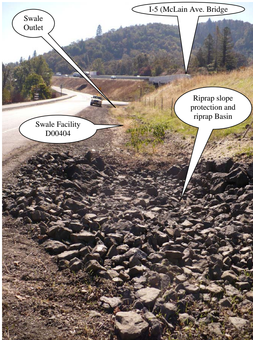
Photo 3: Photo looking south at the 185 ft. swale with inlet shown at the bottom of picture and outlet shown at the top of the picture.
