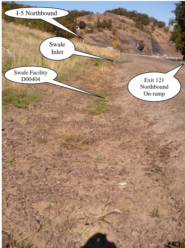
Photo 1: Looking north at the 185 ft. swale from the outlet. Flow into this swale is generated from I-5 on the left side of the picture and is diverted into the riprap basin shown at the swale inlet.
