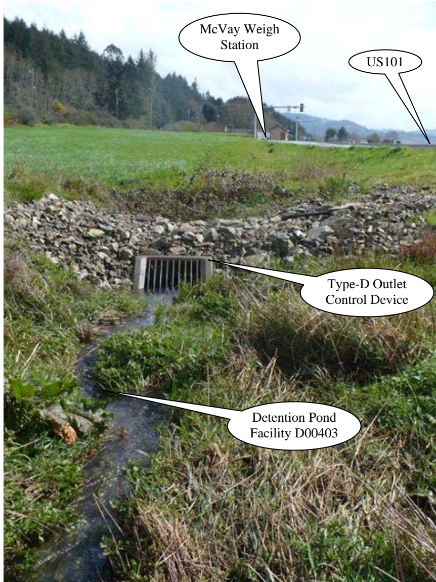
Photo 1: Looking south, stormwater is flowing from the bottom of the picture towards into the outlet control device, shown. During High flow events stormwater will be detained in the pond and released at a controlled rate through a 6-inch pipe located in the Type-D inlet.
