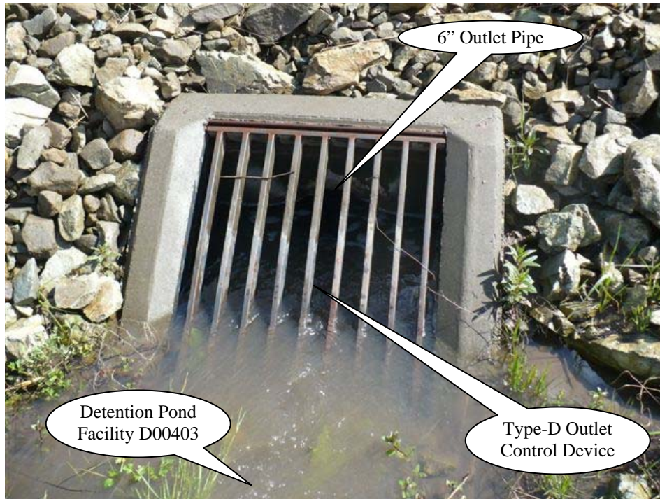
Photo 3: Looking south, stormwater is flowing from the bottom of the picture towards into the outlet control device, shown. During High flow events stormwater will be detained in the pond and released at a controlled rate through a 6-inch pipe located in the outlet control device.
