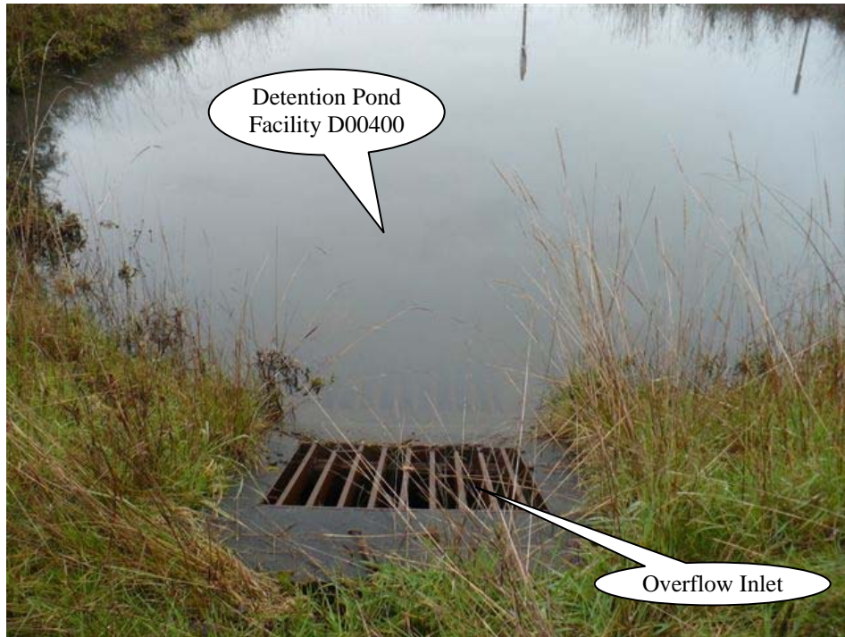
Photo 2: Type-D overflow inlet allows the free discharge of stormwater during high flow events.
