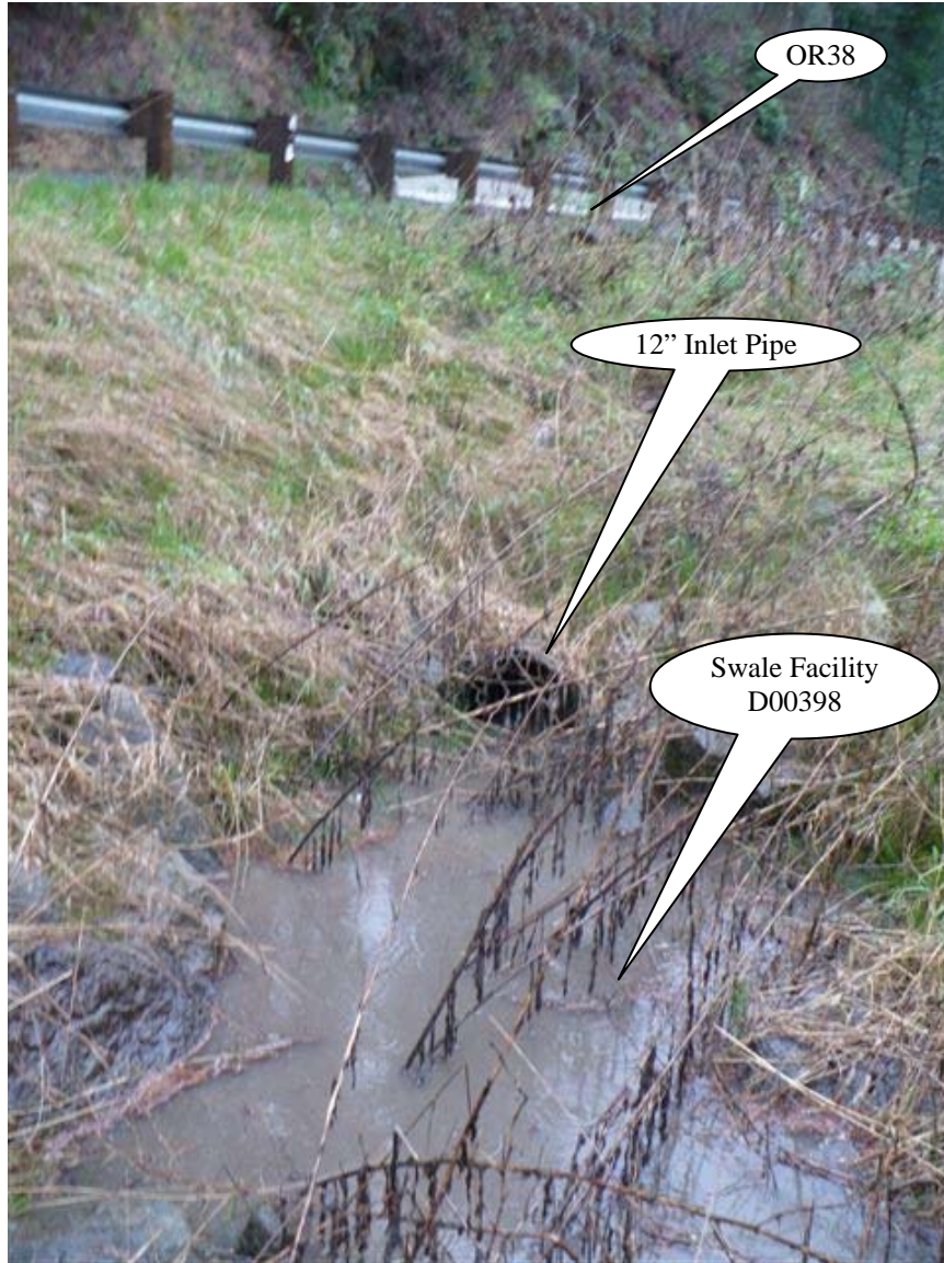
Photo 2: Looking west, storm flow generated from OR38 on the left side of the picture contributes stormwater into the swale. The 12-inch inlet pipe shown contributes storm flow from the Elk Creek Bridge.
