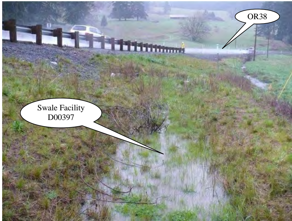
Photo 1: Looking east, storm flow generated from OR38 on the left side of the picture contributes stormwater into the swale. Stormwater is flowing from the top of the picture towards the bottom of the picture.
